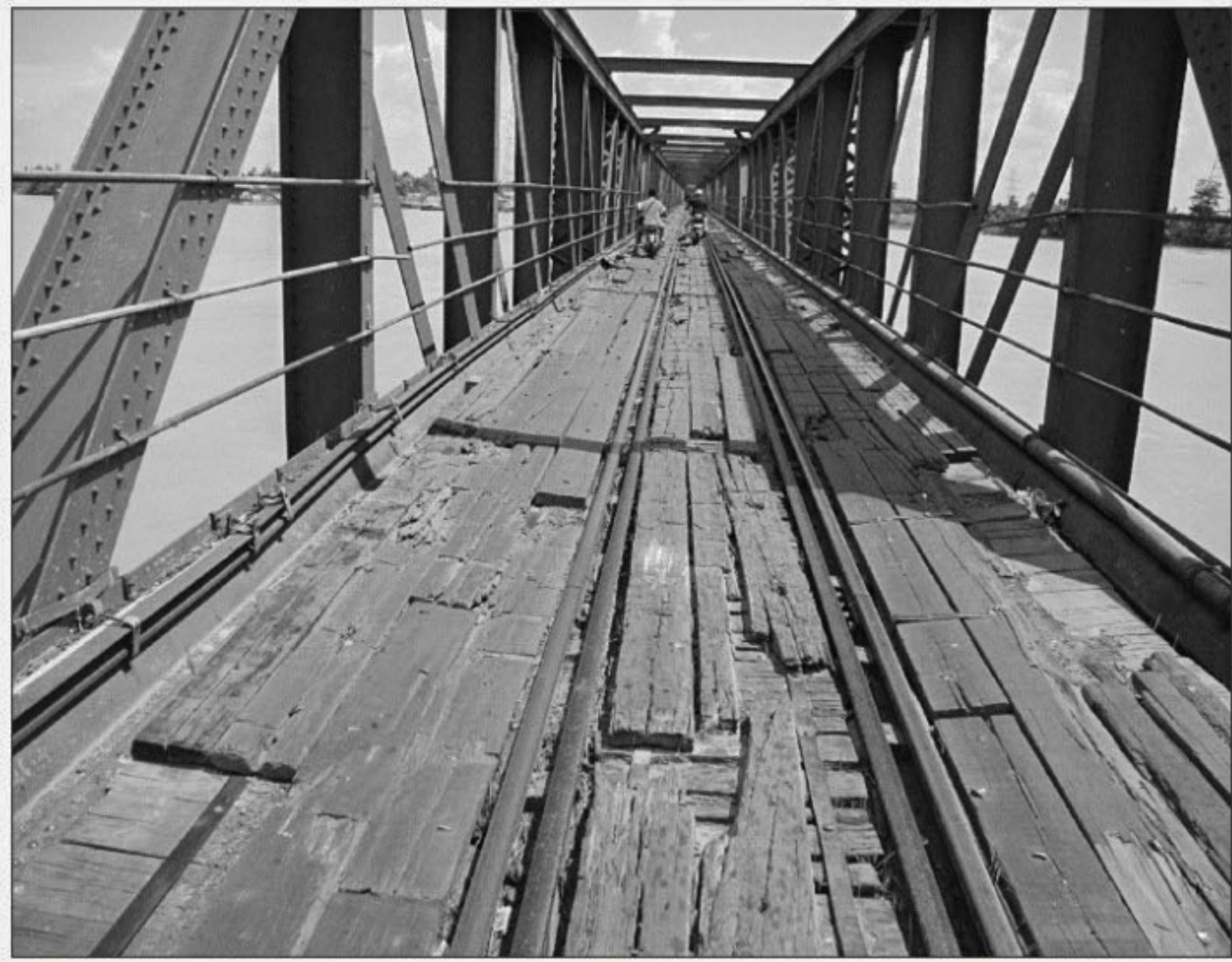
PHOTO: STAR This time-expired railway-cum-road bridge over the Teesta River in Lalmonirhat Sadar upazila has turned awfully risky as the wooden floorboards, set in 1978 to facilitate movement of light vehicles, have weakened due to plying of heavy vehicles.
