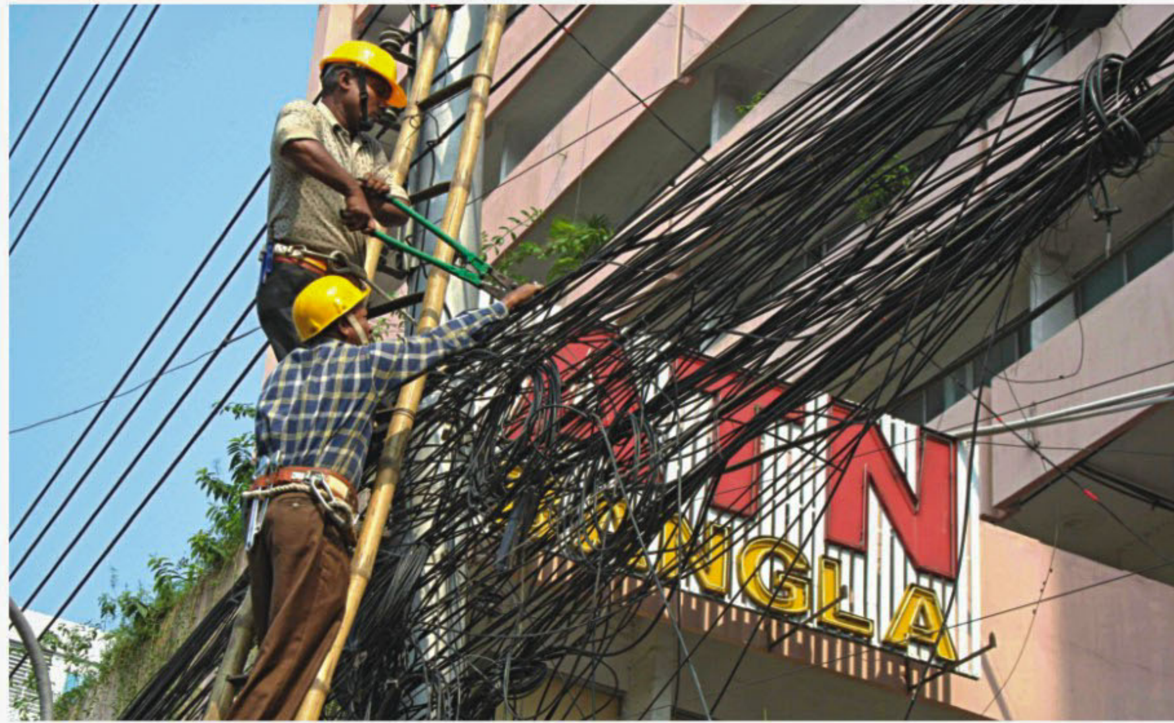
Government workers remove the tangle of internet and cable TV wires hanging from utility poles at Karwan Bazar in the capital yesterday disrupting internet service and cable TV service to many homes and organisations. PHOTO: STAR
