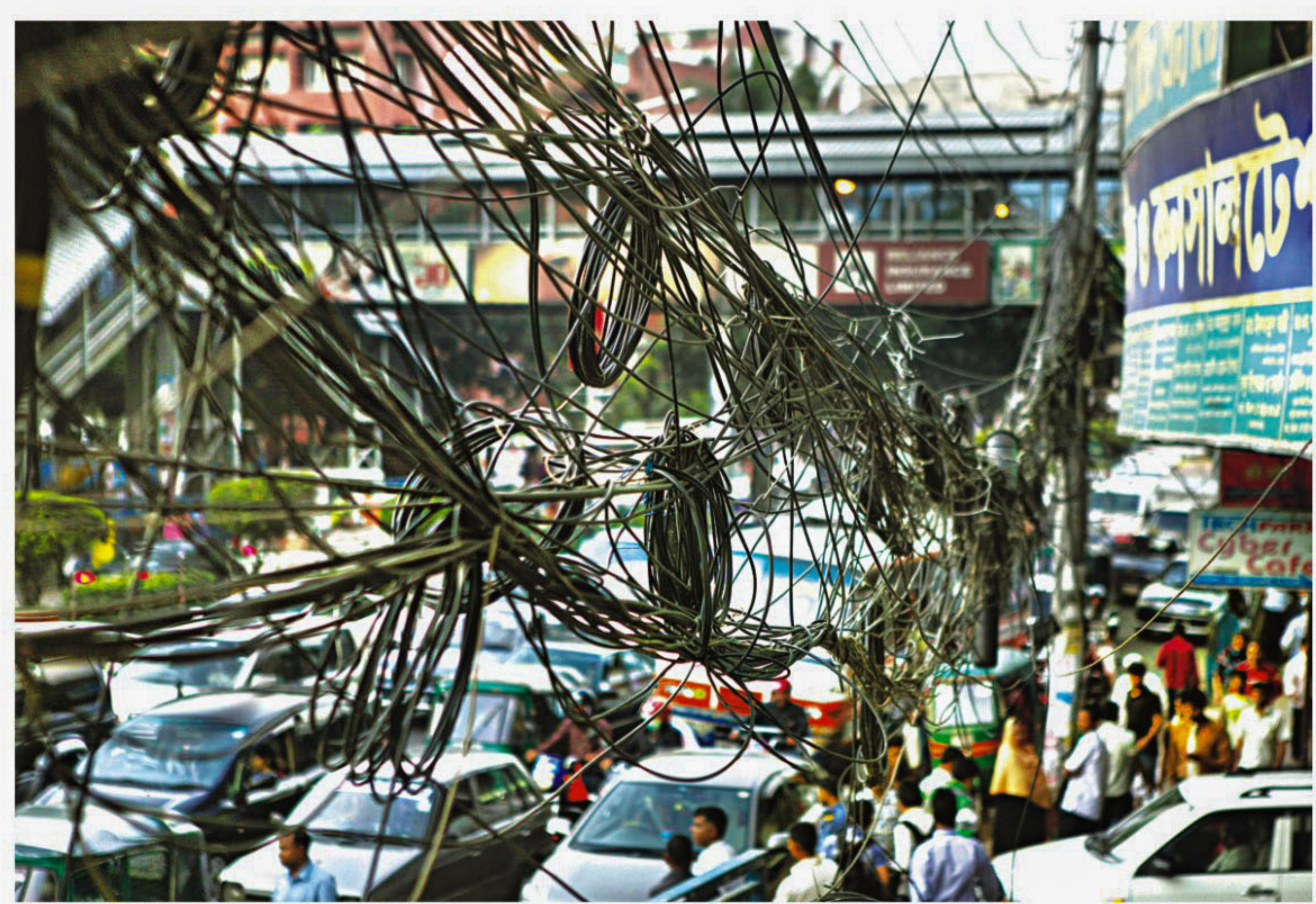
The tangle of wires at Farmgate is likely to be removed today as a government drive begins on all overhead Internet and cable TV wires on thoroughfares between Uttara and Shahbagh. PHOTO: STAR
