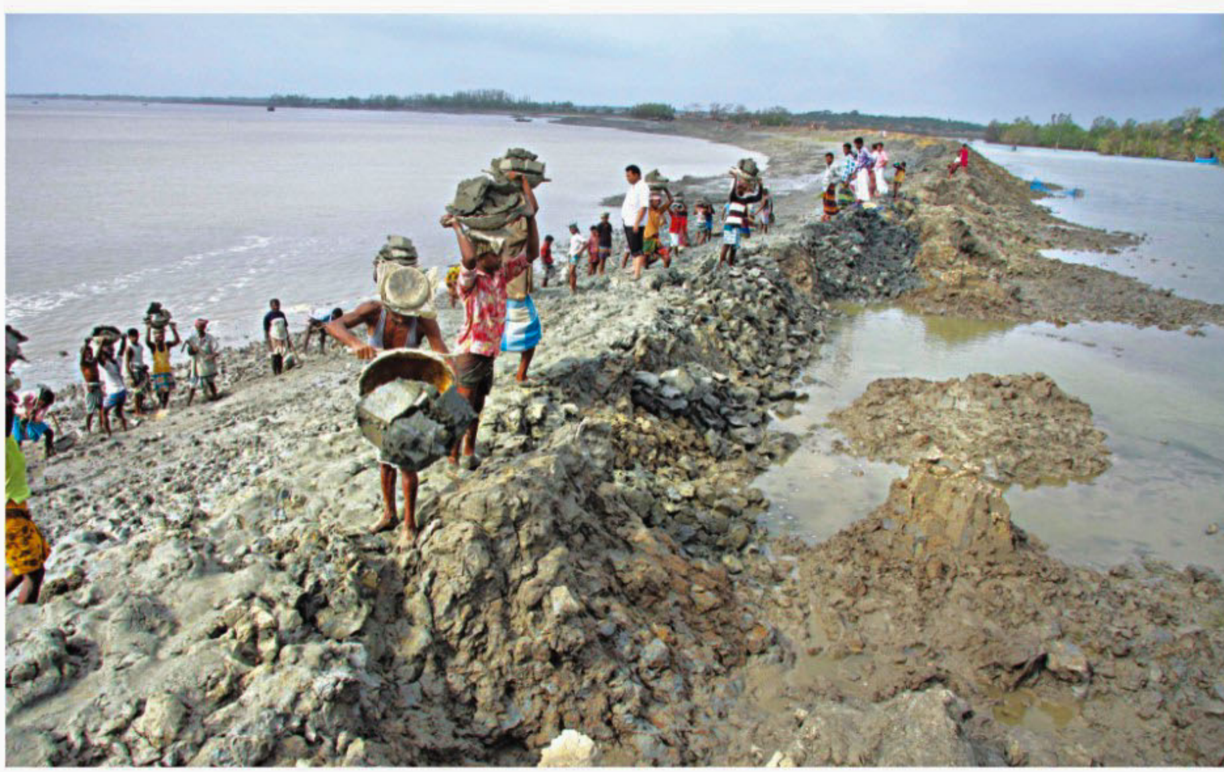
Locals at Gabura in Satkhira rebuild an embankment ravaged by Aila last year that caused woes for millions.
