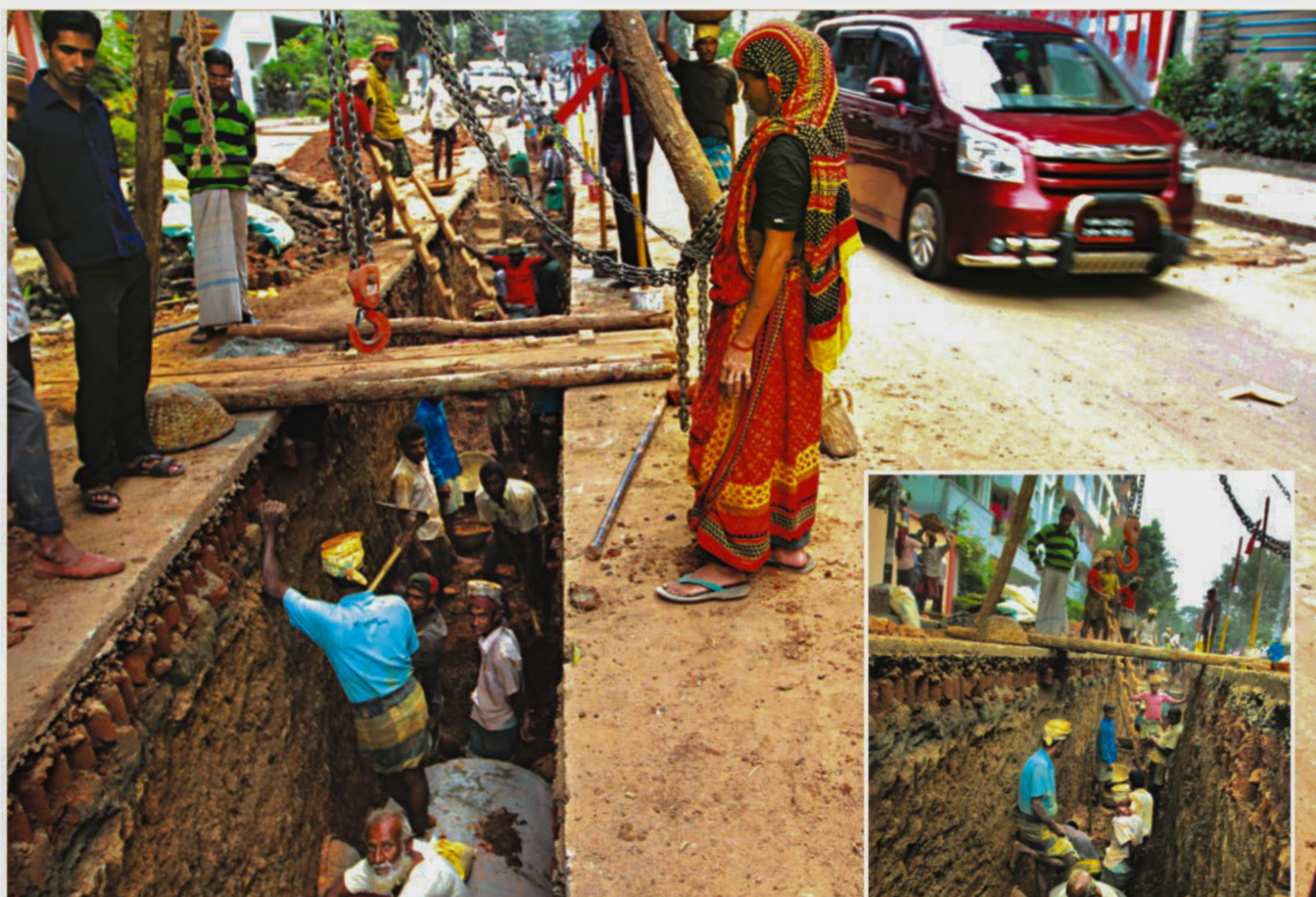
Dhaka Wasa is digging up roads in different parts of the city to install drainage pipes causing sufferings to the dwellers. These photos were taken from Dhanmondi, Road No 8.
