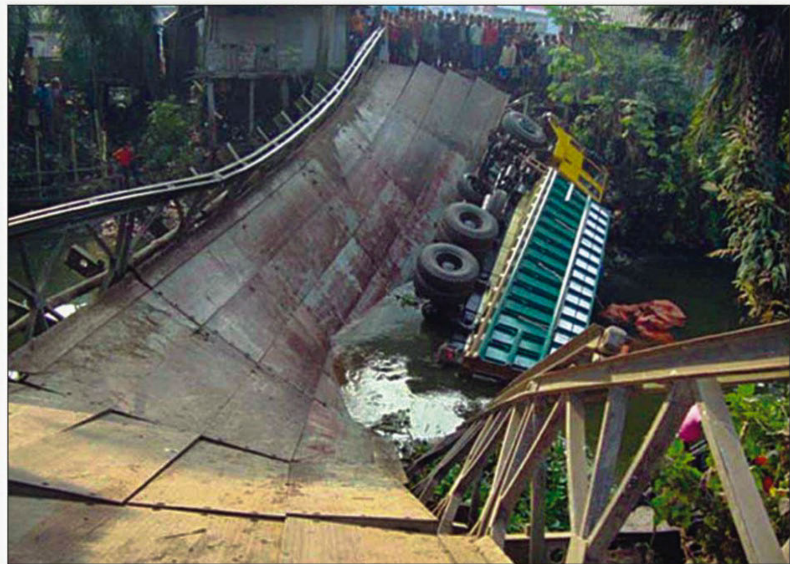
This bailey bridge over Chitra River at Chitalmari in Bagerhat district collapsed under the pressure of a stone-laden truck on Sunday.
