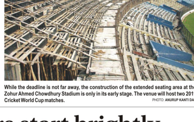
While the deadline is not far away, the construction of the extended seating area at the Zohur Ahmed Chowdhury Stadium is only in its early stage. The venue will host two 2011 Cricket World Cup matches.
