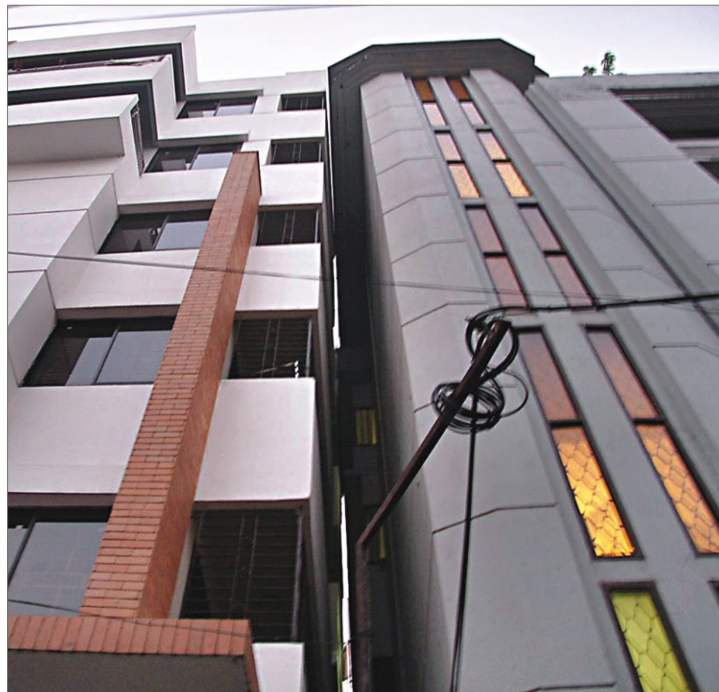
The building 'Chand Nibash', left, has tilted towards the adjoining six-storied 'Reliance Plaza' in Chittagong Development Authority (CDA) residential area of Agrabad in the port city yesterday.
