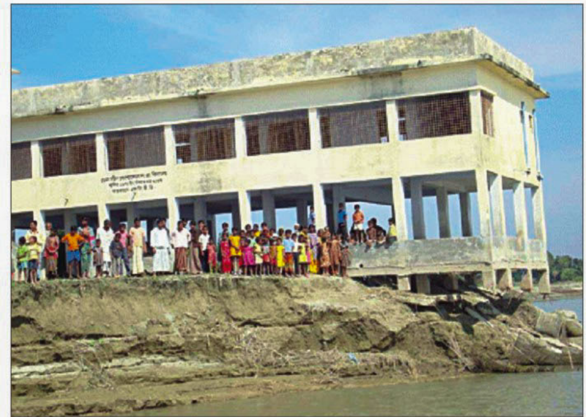
Dakhhin Char Panchakola Primary School in Bera upazila of Pabna district remains in an awfully dangerous condition as a portion of the ground under the building has moved away due to erosion by the Jamuna.
