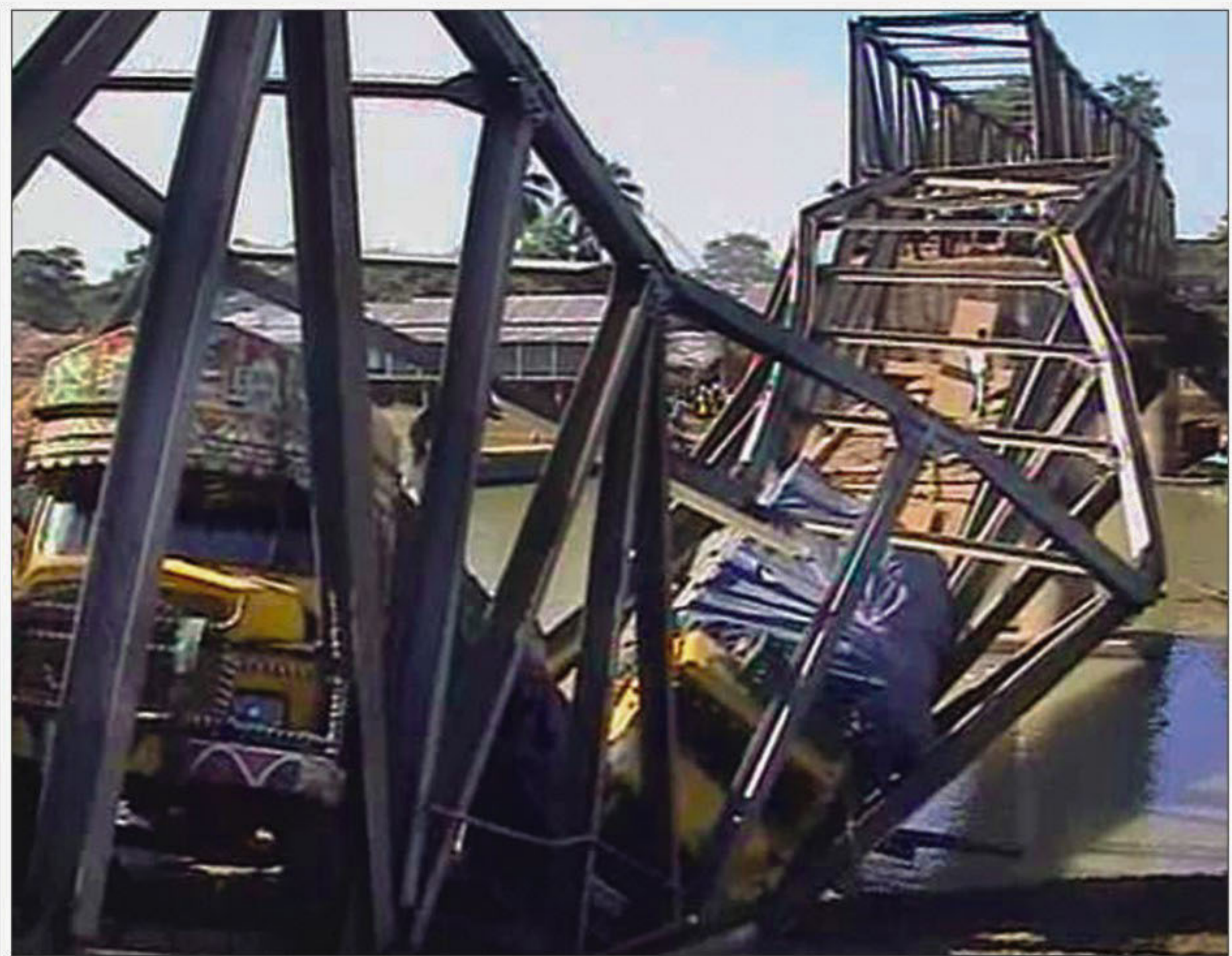
Left in a decrepit condition for long, this bailey bridge at Thakurakona on Netrakona-Mohanganj road collapsed under the pressure of a truck yesterday.
