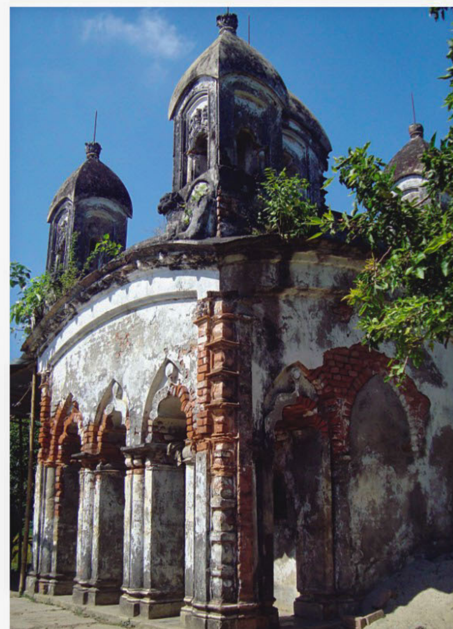
Grass and plants have sprouted on the temple's walls and roof, while cracks have developed around the structure.
