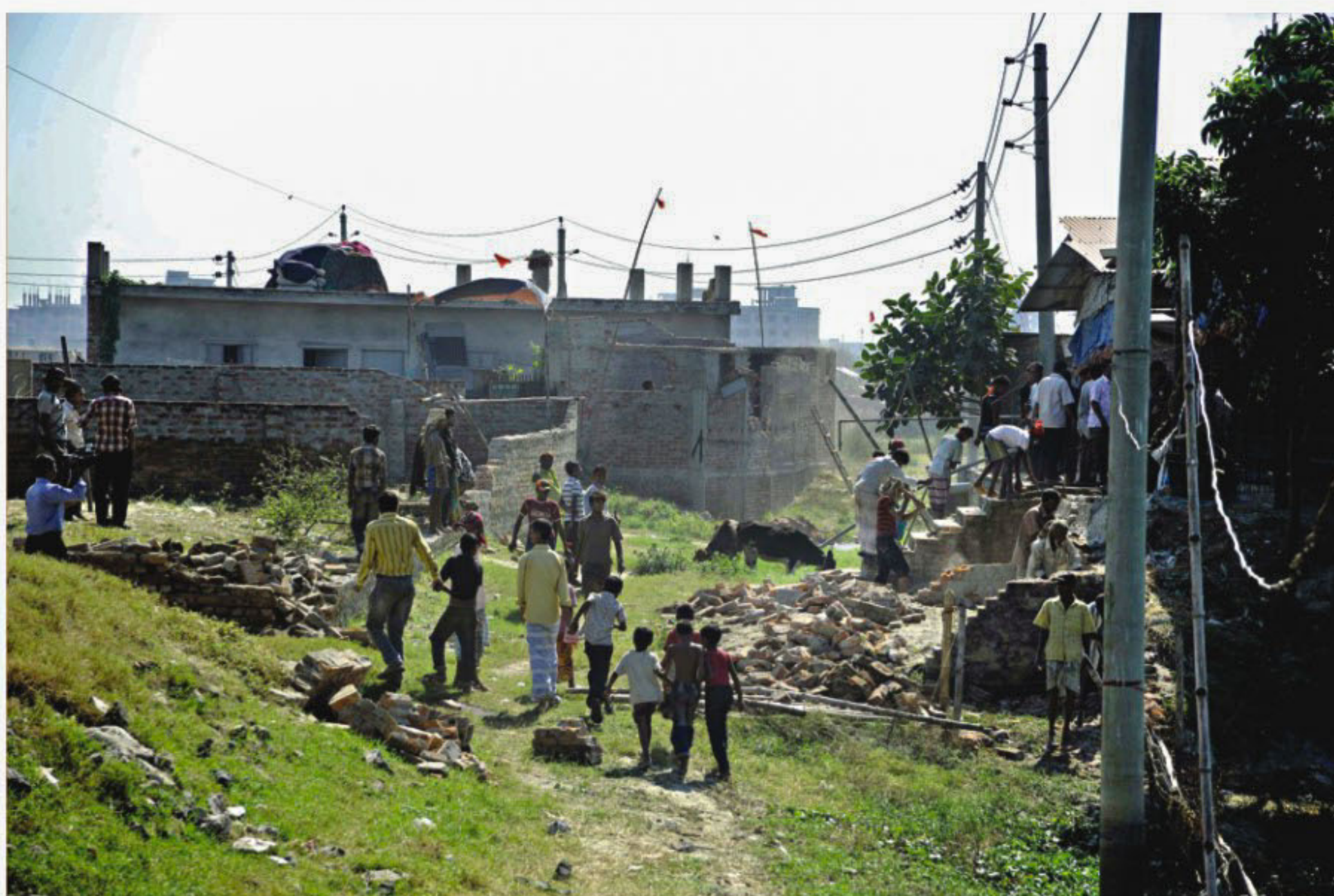
Dhaka Wasa, with the assistance of local lawmaker, and the district administration conduct a joint drive to dismantle illegal structures on a Kalyanpur canal yesterday. Attempts like these receive much praise but encroachers eventually return after some time. PHOTO: STAR
