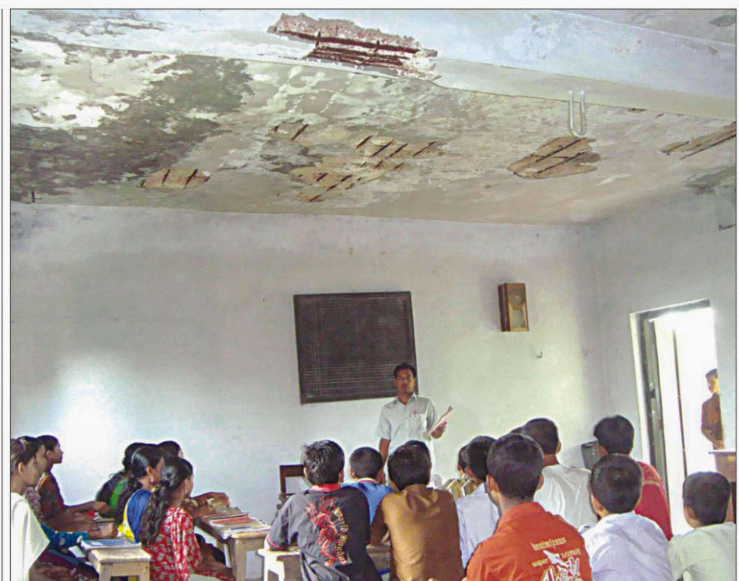
Students attend their class under the decrepit roof of century-old Raigram High School in Kaliganj upazila of Jhenidah district.
