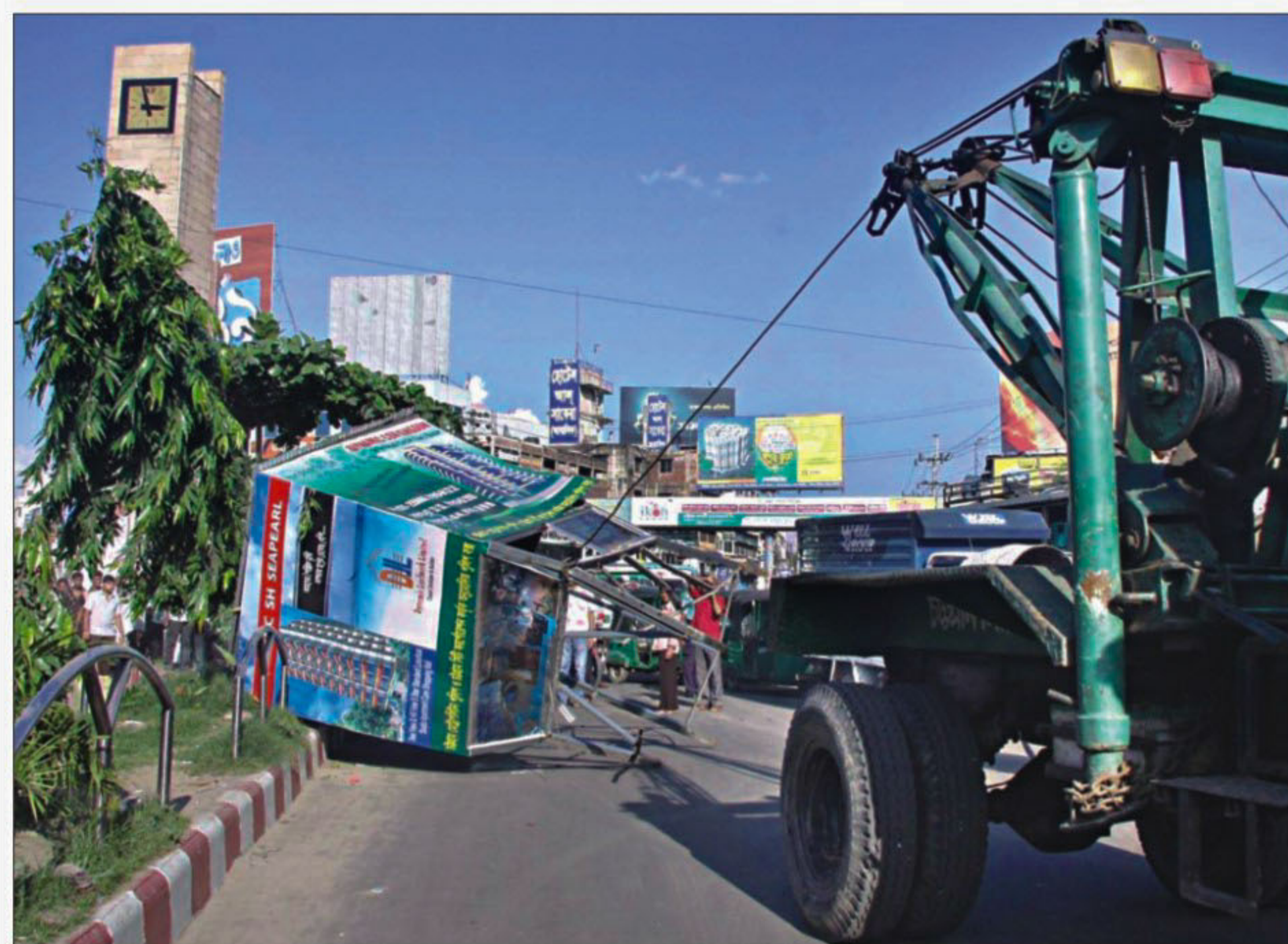
Chittagong City Corporation (CCC), in a drive, knocks down an illegal police box at Bahoddarhat crossing in the port city yesterday. The CCC removed seven more police boxes from the city on the day.
