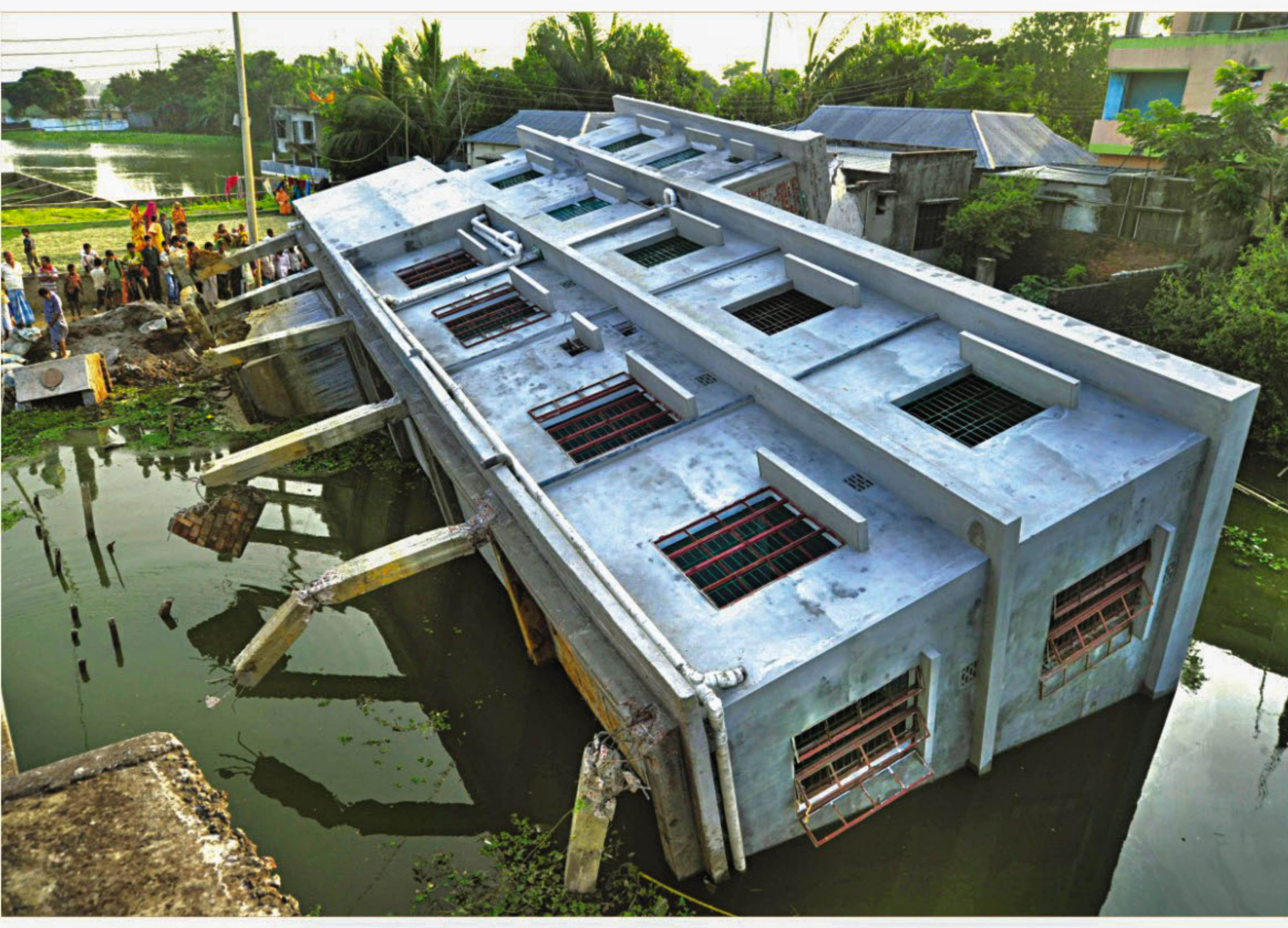
This newly built three-storey building in a jheel at Norda, Dakhinkhan collapsed on a tin-roof house Tuesday night.
