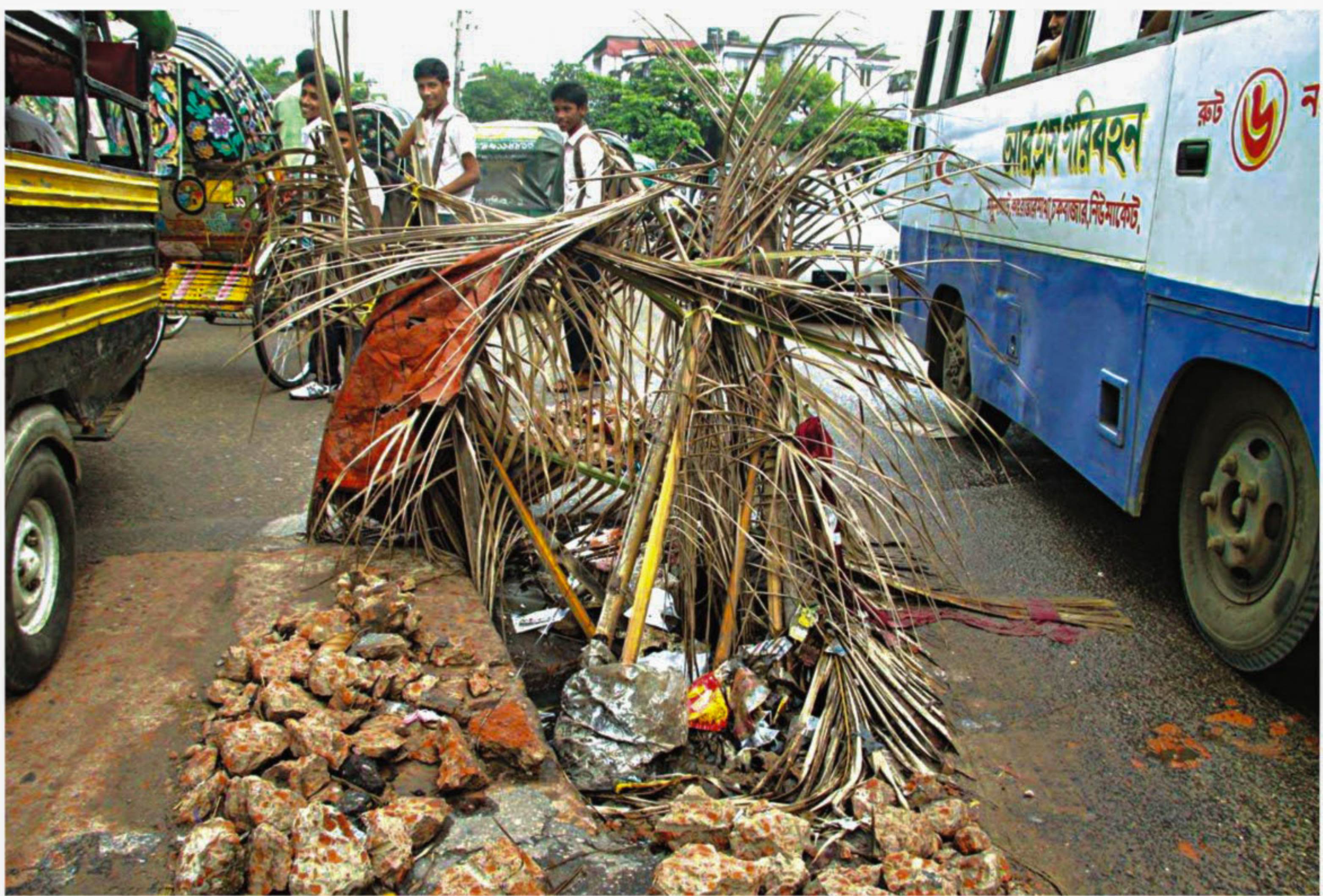
Locals put leaves and branches into the manhole to signal to people that its lid is broken. The open manhole on the main street in Patchlish-Katalganj area in the port city causes accidents almost every night.
