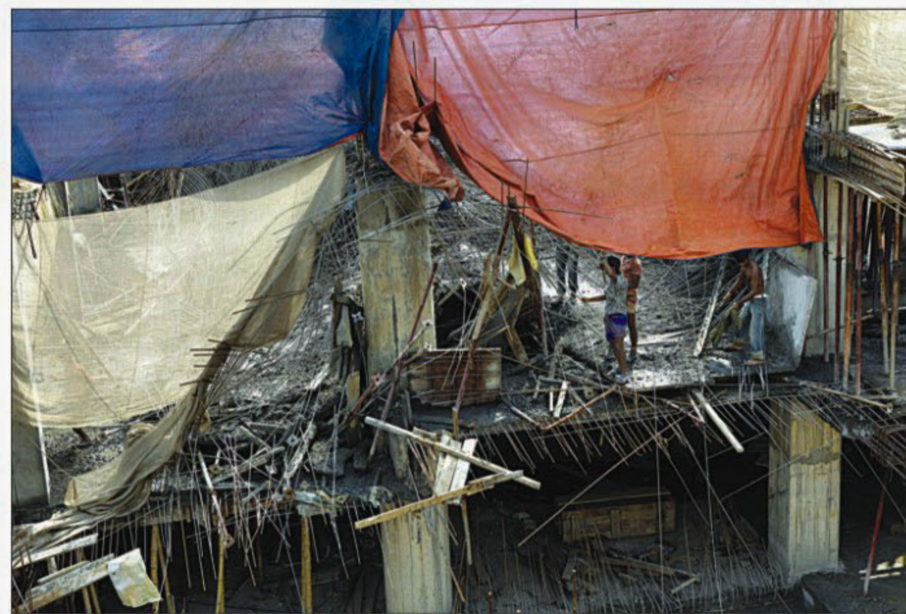
A portion of the first floor of the under-construction Navana Zohura Square building that collapsed at Bangla Motor in the city yesterday morning.
