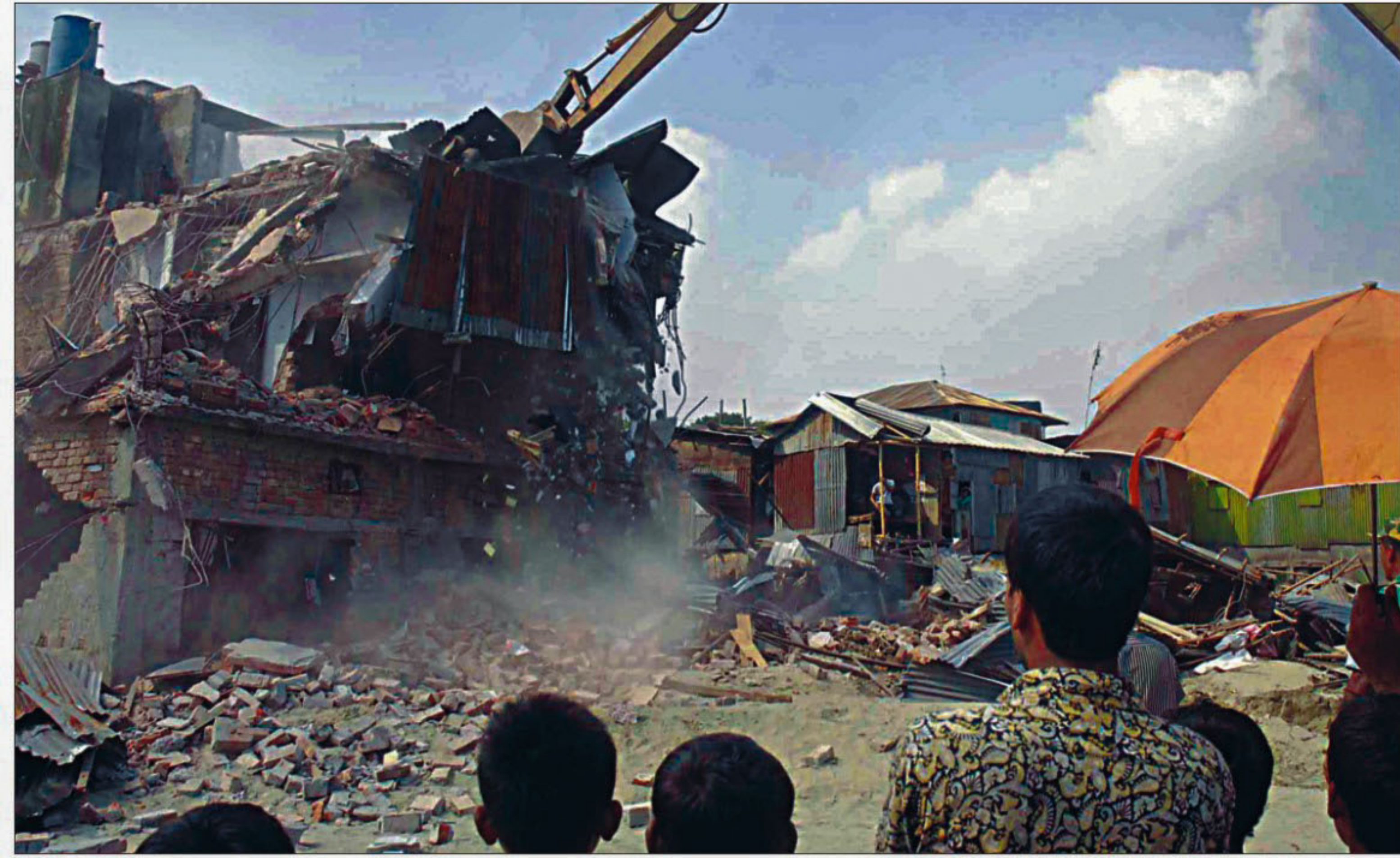
Rajuk demolishes the illegal buildings in Hatirjheel area on Begunbari Khal (canal) in the city yesterday. The drive began on Tuesday.
