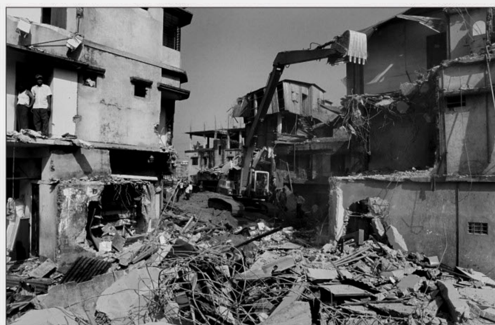
Rajuk knocks down illegal structures constructed on the sideline of Begunbari-Hatirjheel development project yesterday.
