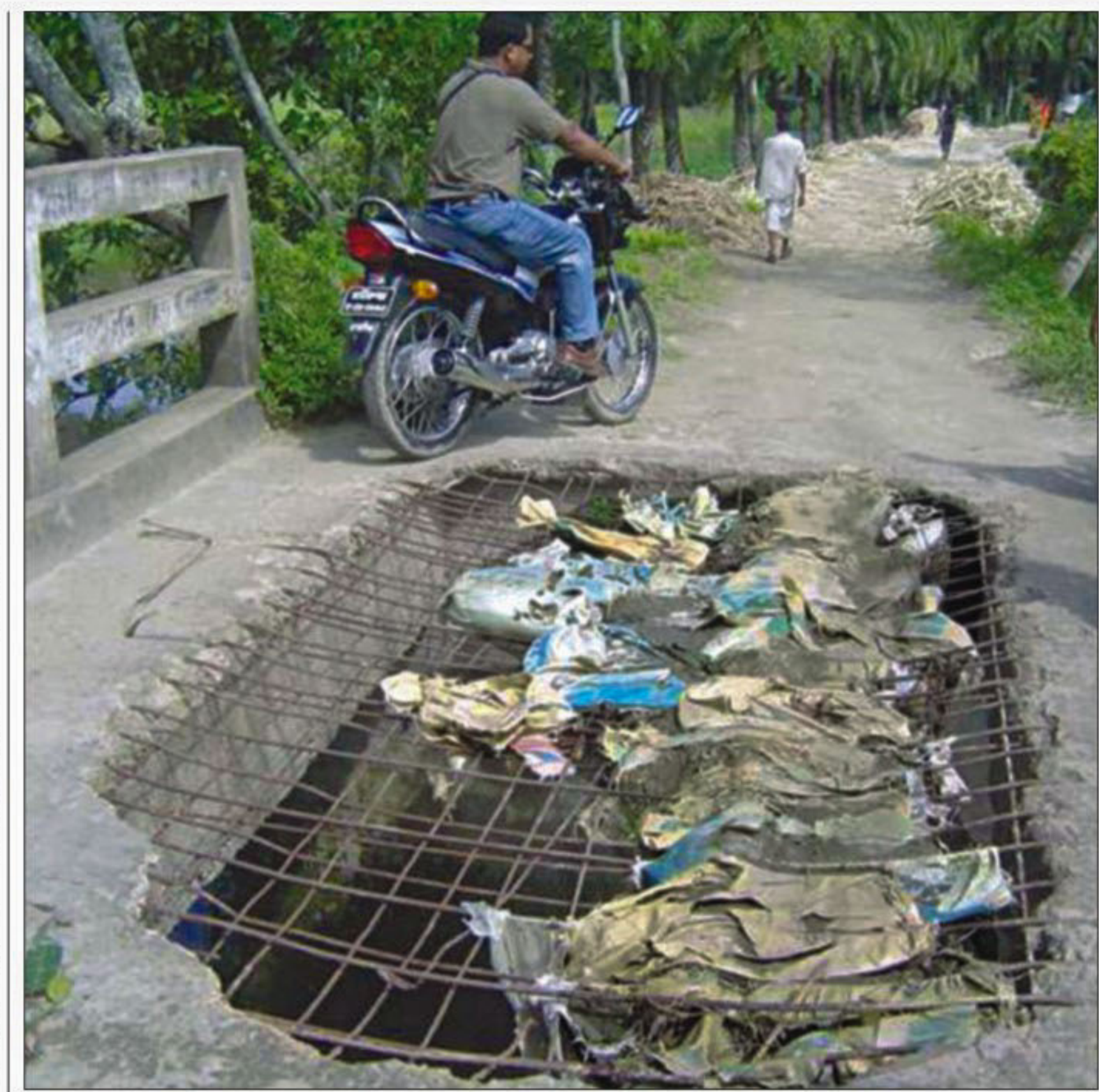
PHOTO: STAR This bridge on Machain-Jhitka road in Harirampur of Manikganj has remained in a dilapidated condition, off-limiting movement of heavy vehicles and posing serious risk for pedestrians and bike riders.
