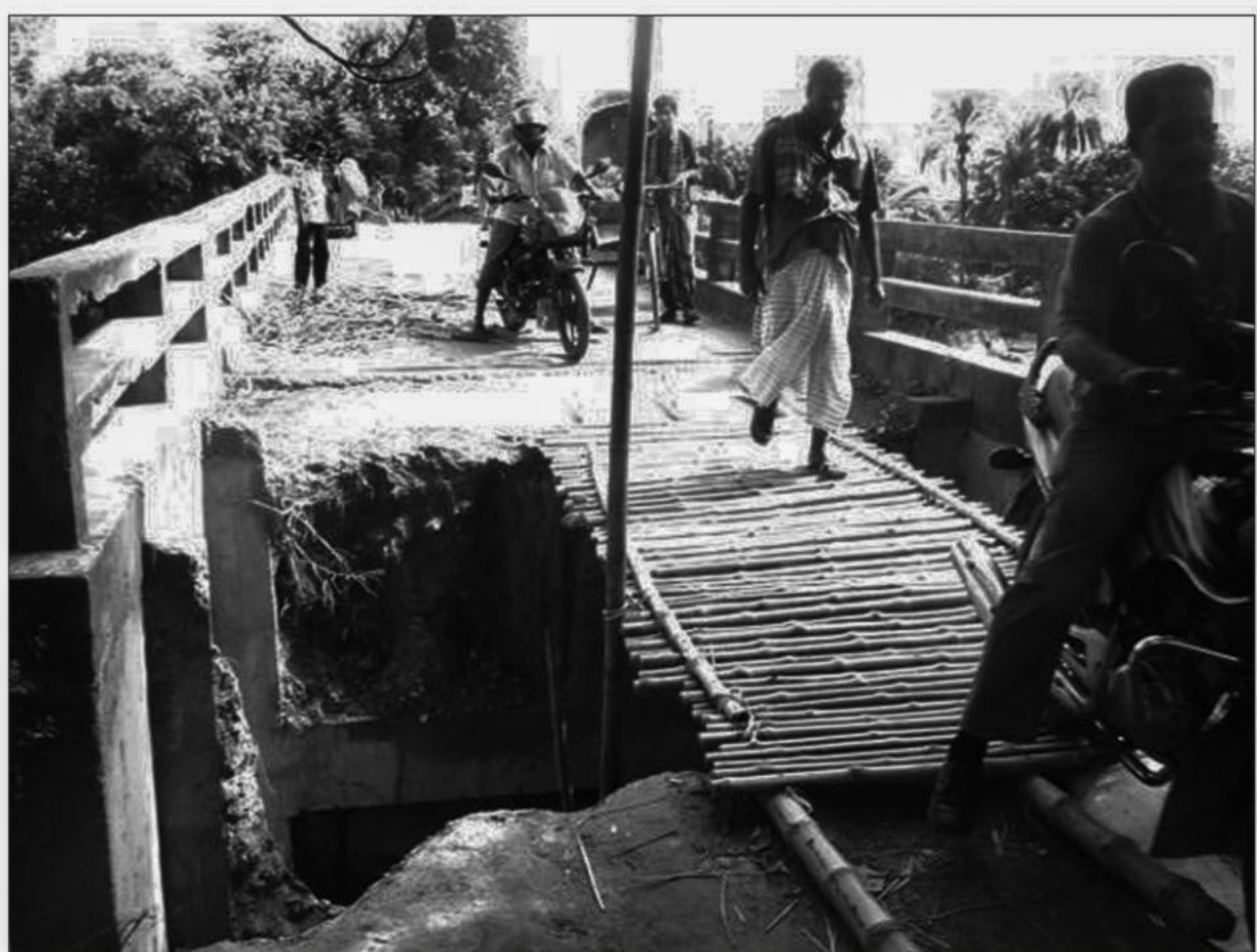
Pedestrians, rickshaws and motorcycles move amid risk through the bamboo-made link of Gangasagar bridge on Aricha-Harirampur road while the area has remained off-limits to buses and cars as the approach road of the bridge has collapsed.
