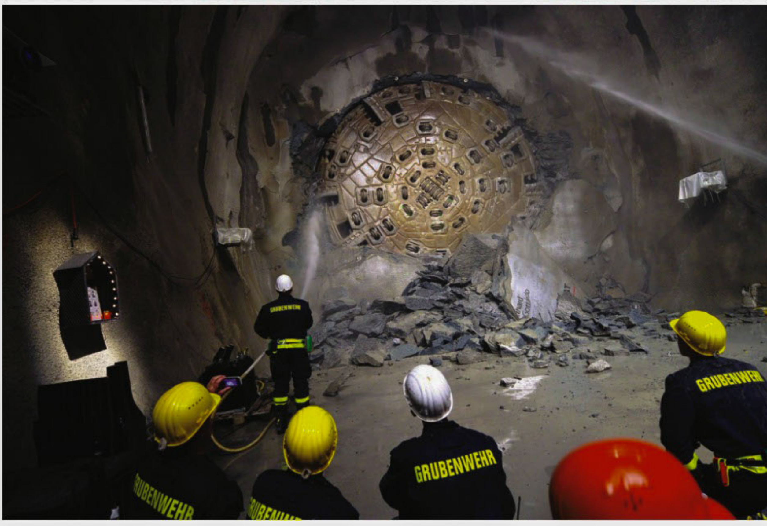
A giant drilling machine completes the world's longest tunnel beneath the Swiss Alps during a ceremony yesterday 30 kilometres from one end and 2,000 metres below the mountains. PHOTO: AFP
