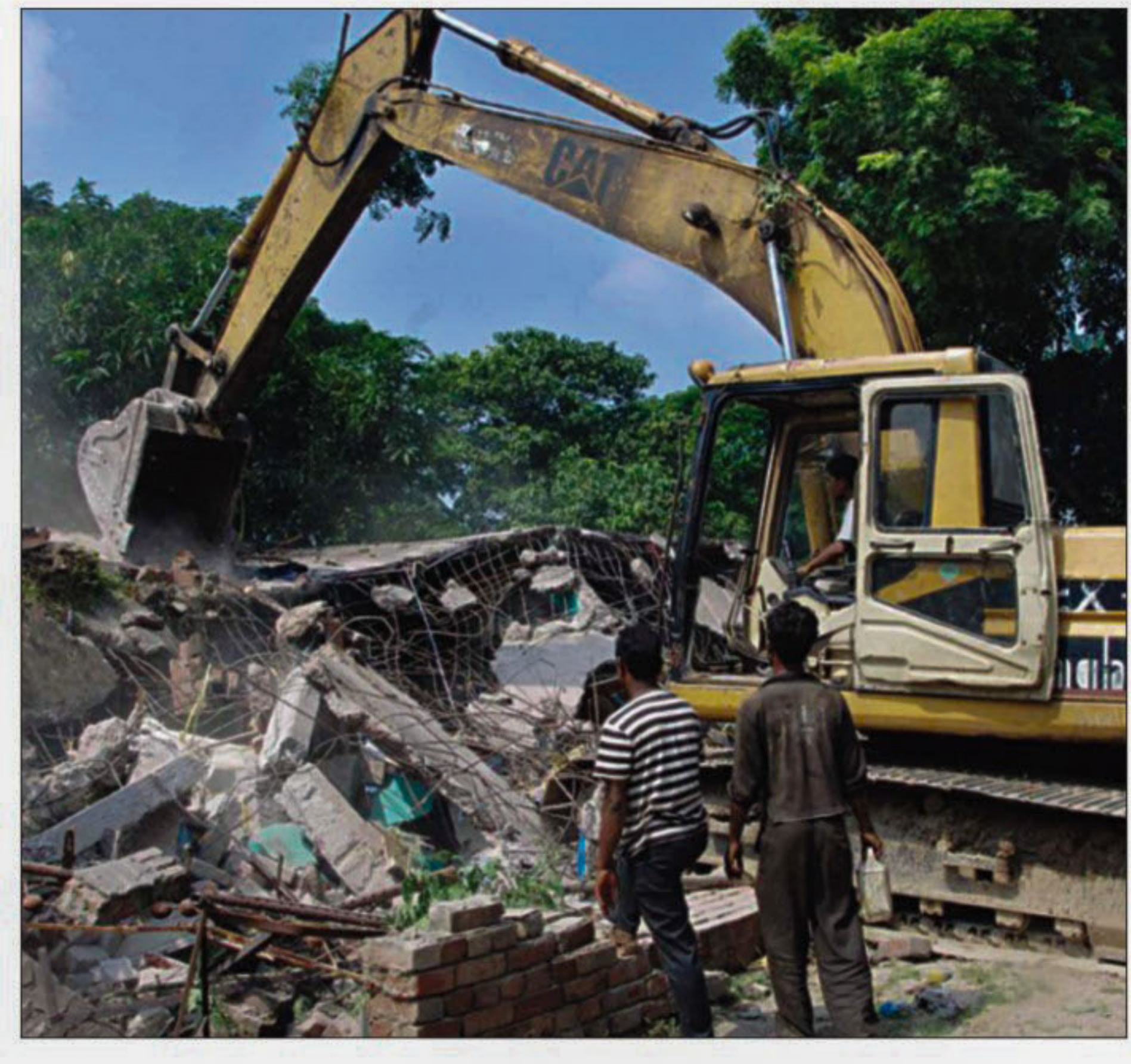
A bulldozer demolishes an illegal structure at Ghoshpara in Rajshahi city yesterday as the city corporation has continued the drive to ease movement of traffic and pedestrians.
