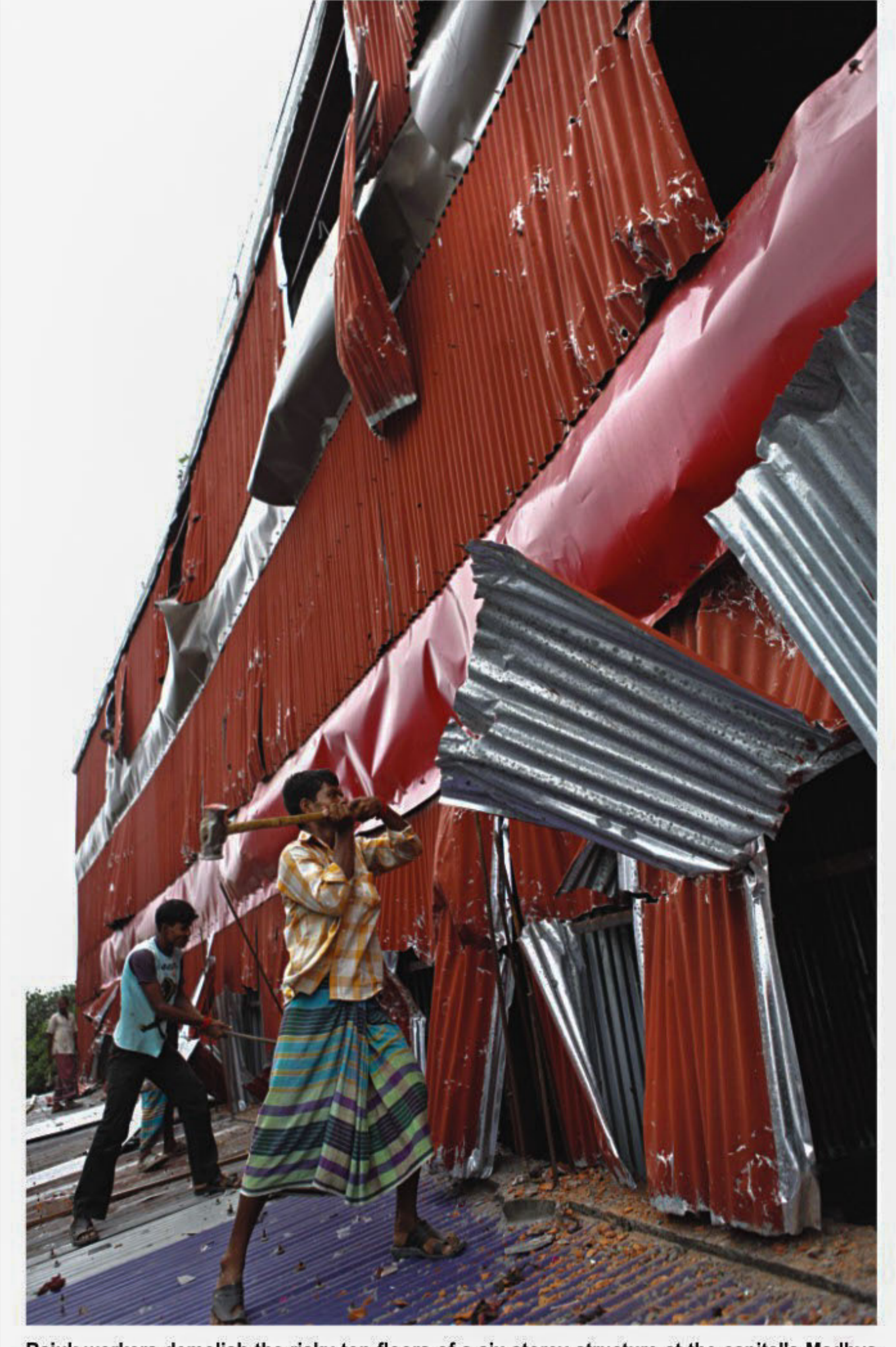
Rajuk workers demolish the risky top floors of a six-storey structure at the capital's Madhya Kunipara in Tejgaon industrial area yesterday.
