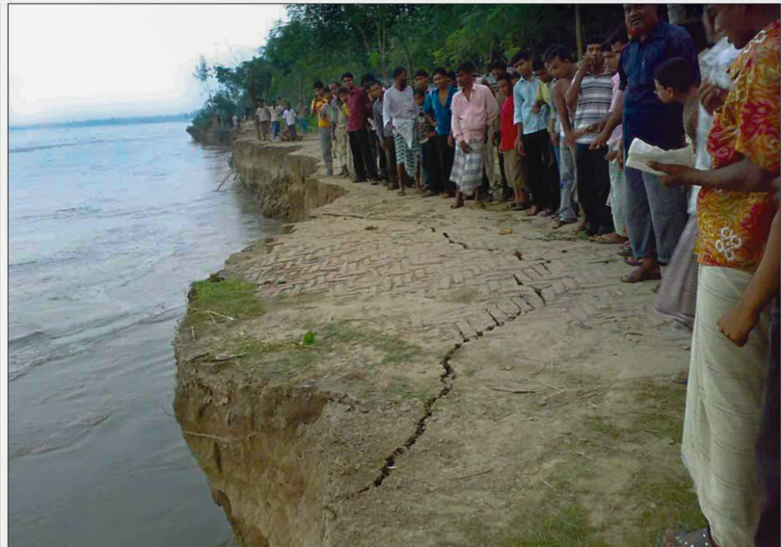
With erosion by the Padma River taking an alarming turn during the last two weeks, this brick-built road at Shara in Pabna district has gone into the riverbed.
