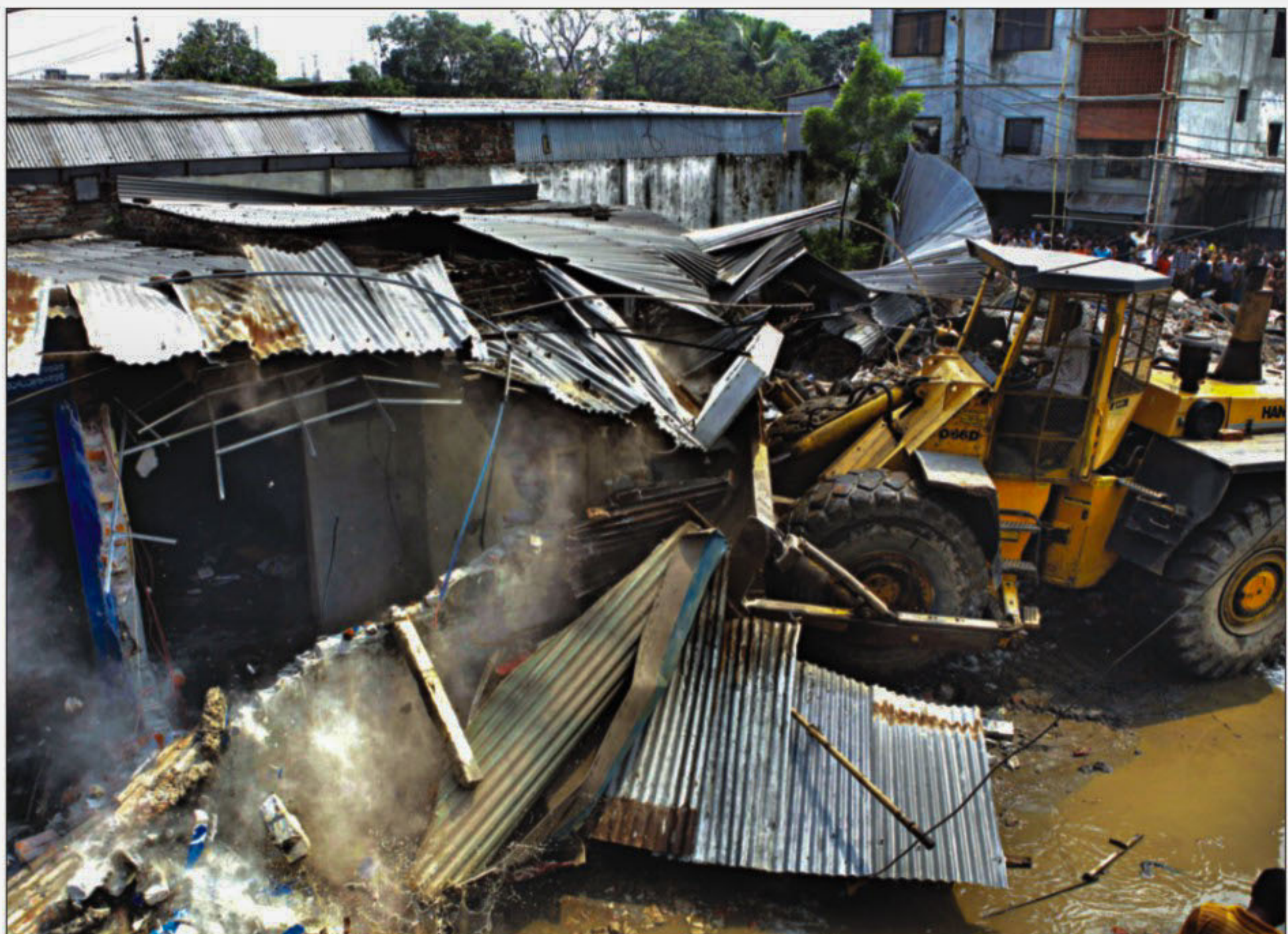
Rajuk demolishes illegal structures at J Block on Road No-20 at Baridhara in the city yesterday.
