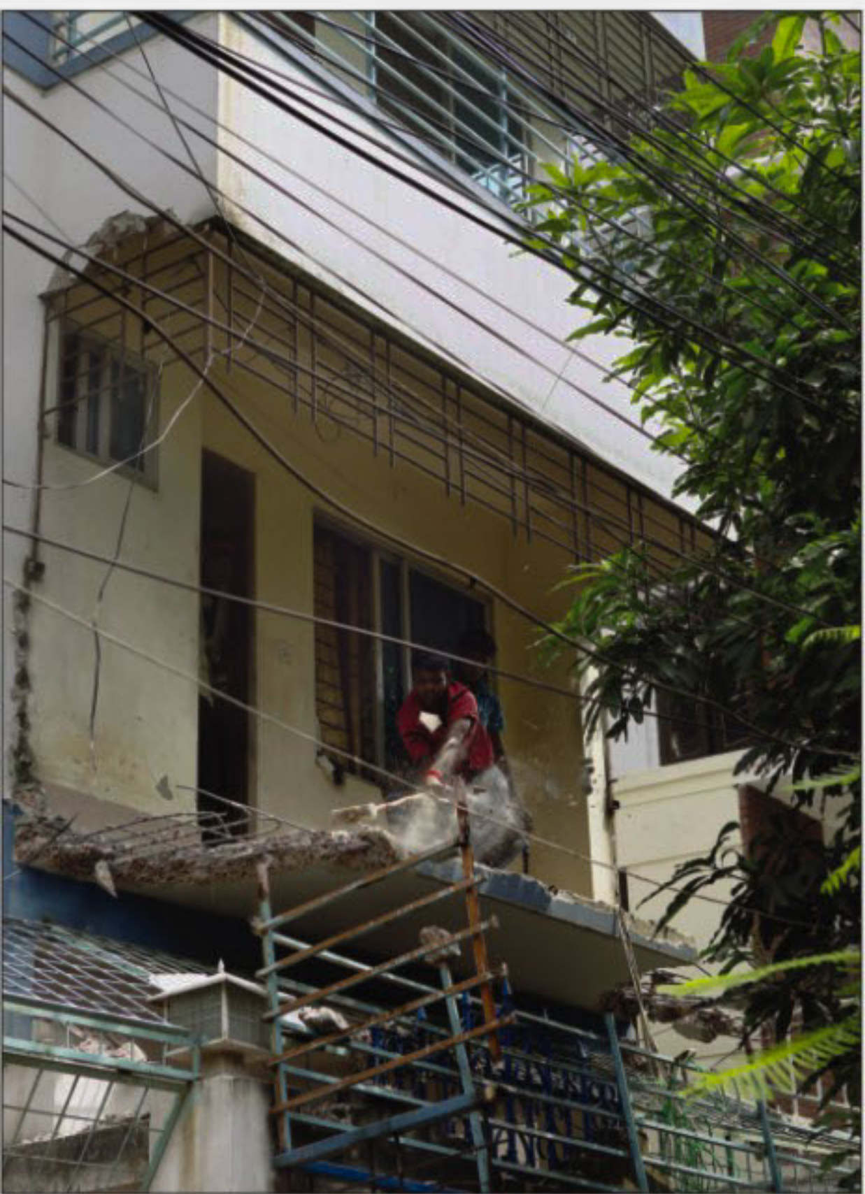
PHOTO: STAR Rajuk dismantles illegal portion of a six-storey building at Uttara Sector No. 3 in the city yesterday.
