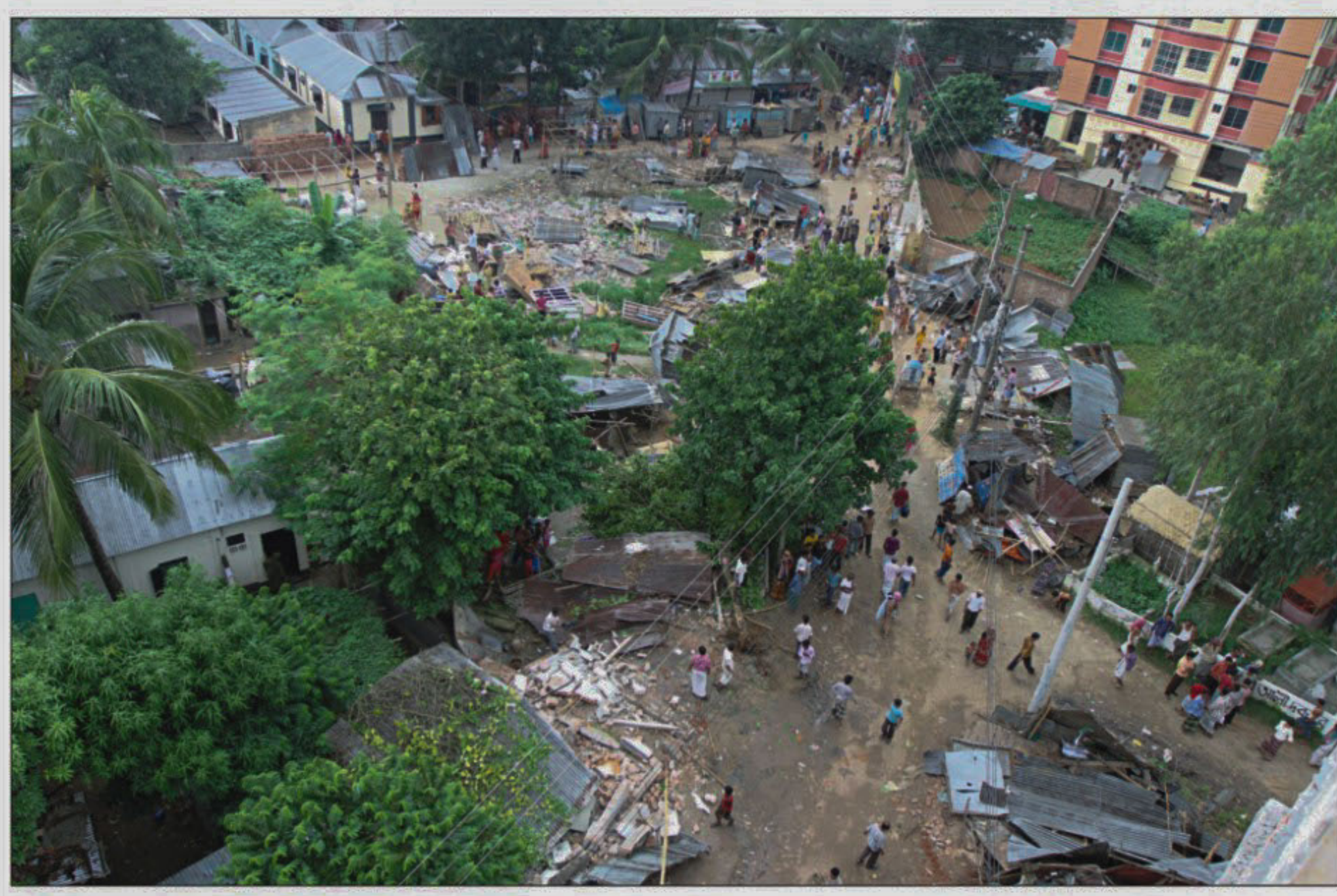
Rajdhani Unnayan Kartripakkha (Rajuk) demolishes illegal structures on Uttara Road No-16-23 near Uttara-Ashulia embankment in the city yesterday. (Story on Page 16)
