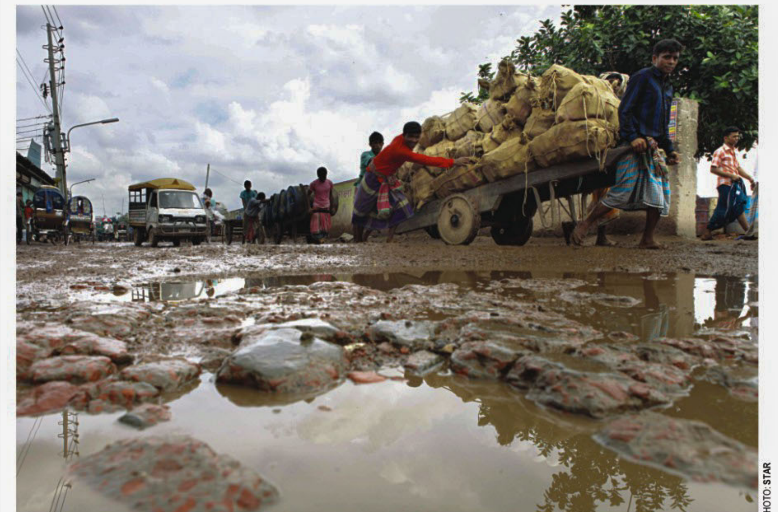
The condition of Gabtoli-Babubazar Road at Sawarighat is simply appalling. The photo was taken early this month. PHOTO: STAR
