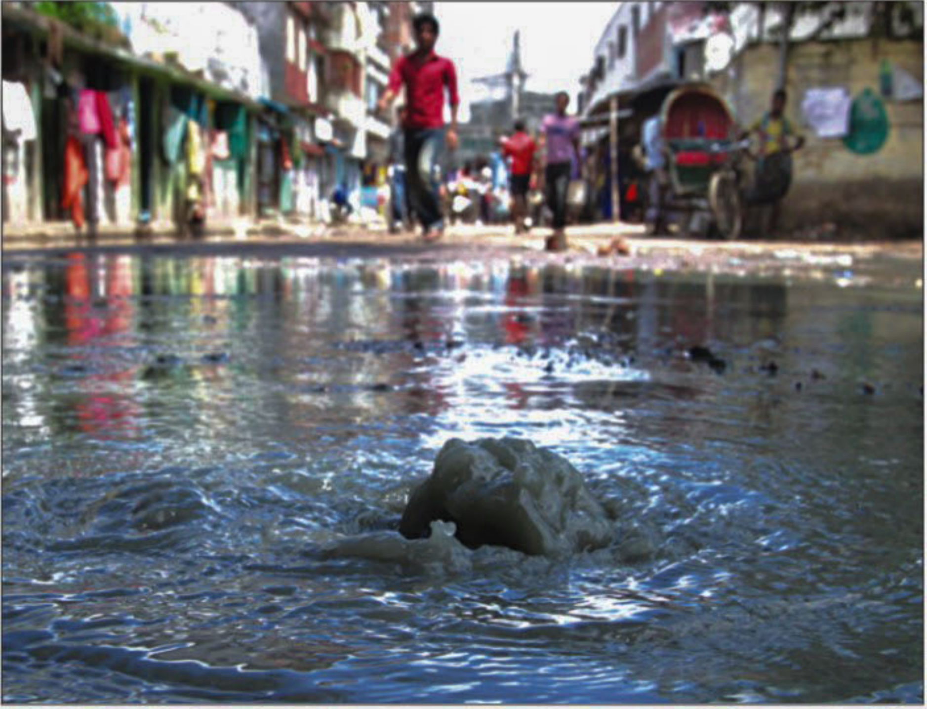
Water from the pipelines of Wasa leaks onto the road at Shashan Ghat Moar in the city's Lalbagh yesterday. The dirty water from sewerage lines also mixes in the water.
