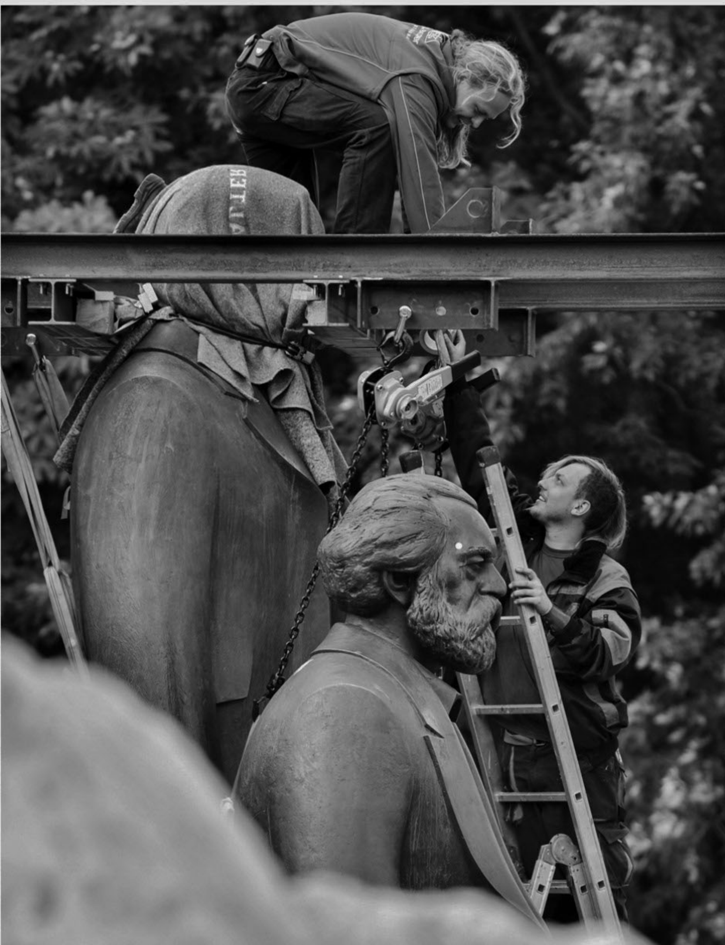
Workers prepare to lift a statue of German political philosopher Friedrich Engels (L) off of its base separating it from a statue of Karl Marx, in Berlin yesterday. The two statues are being moved, one by one to allow for work on the new U55 underground line. They were made by east German sculptor Ludwig Engelhardt and inaugurated in 1986 by then Communist supremo Erich Honecker.
