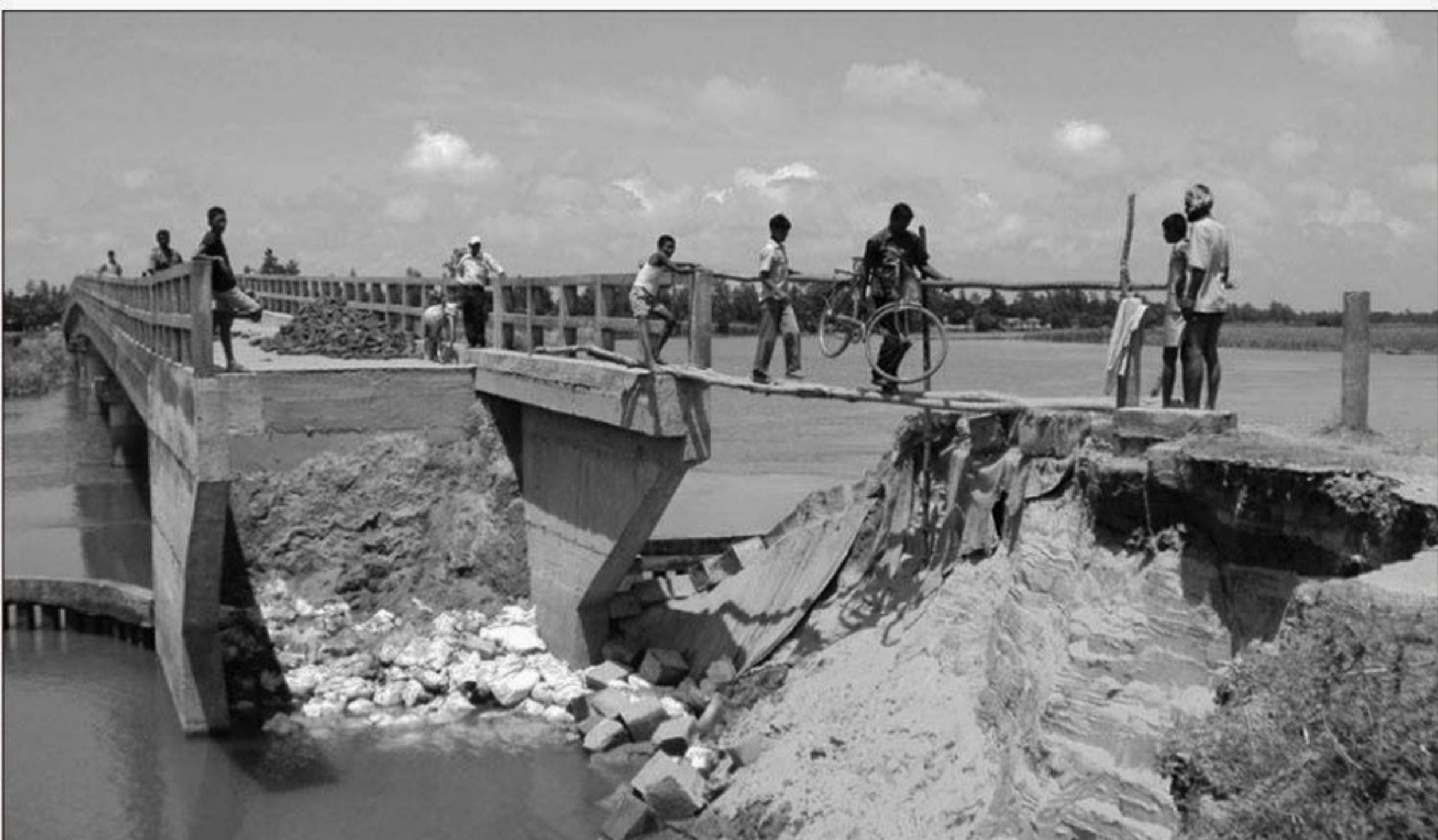
PHOTO: STAR This approach road to Dewantola bridge across Bangali River in Gobindaganj upazila has remained without any repair since its collapse by floodwater on August 28, causing suspension of road communication between Gobindaganj and Saghata upazilas of Gaibandha district.
