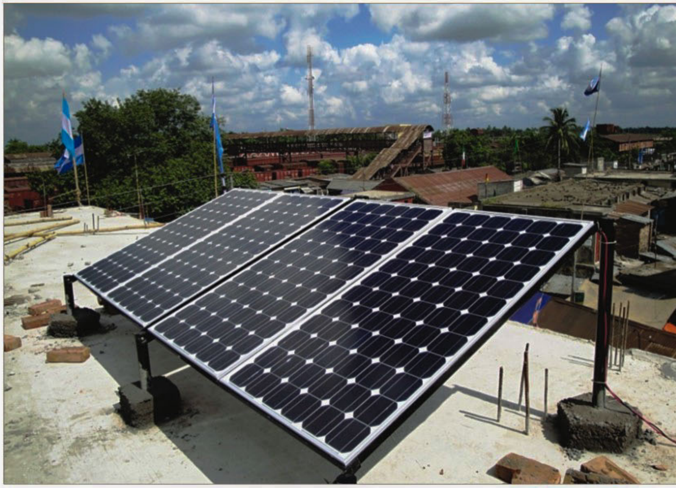
A solar power system installed by Electro Solar in Ishwardi.
