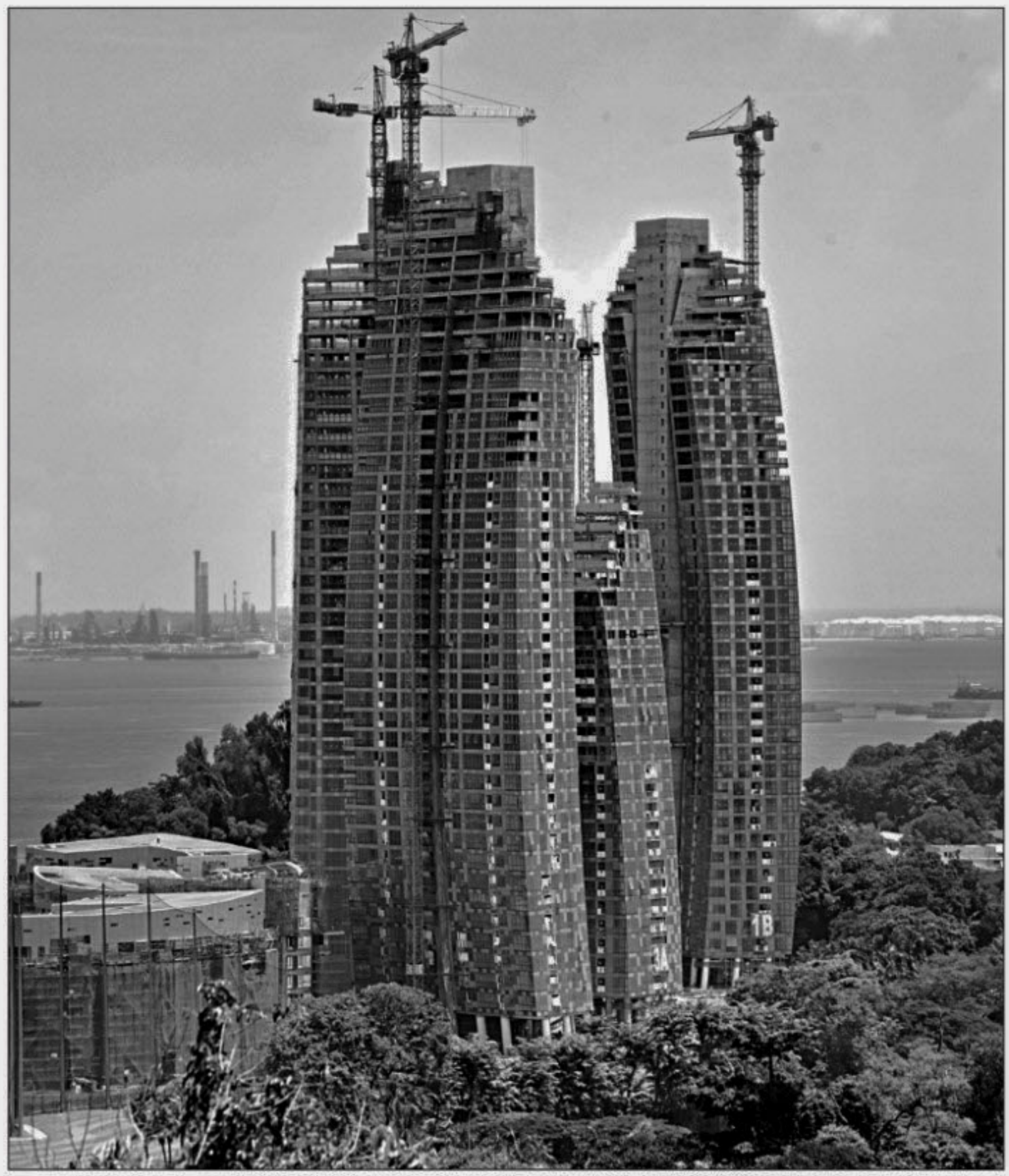
AFP A private condominium under construction near the bay in Singapore is pictured. Asian policymakers fearing a US-style housing market bubble have taken fresh measures to curb runaway property prices as the region leads the global rebound from recession.
