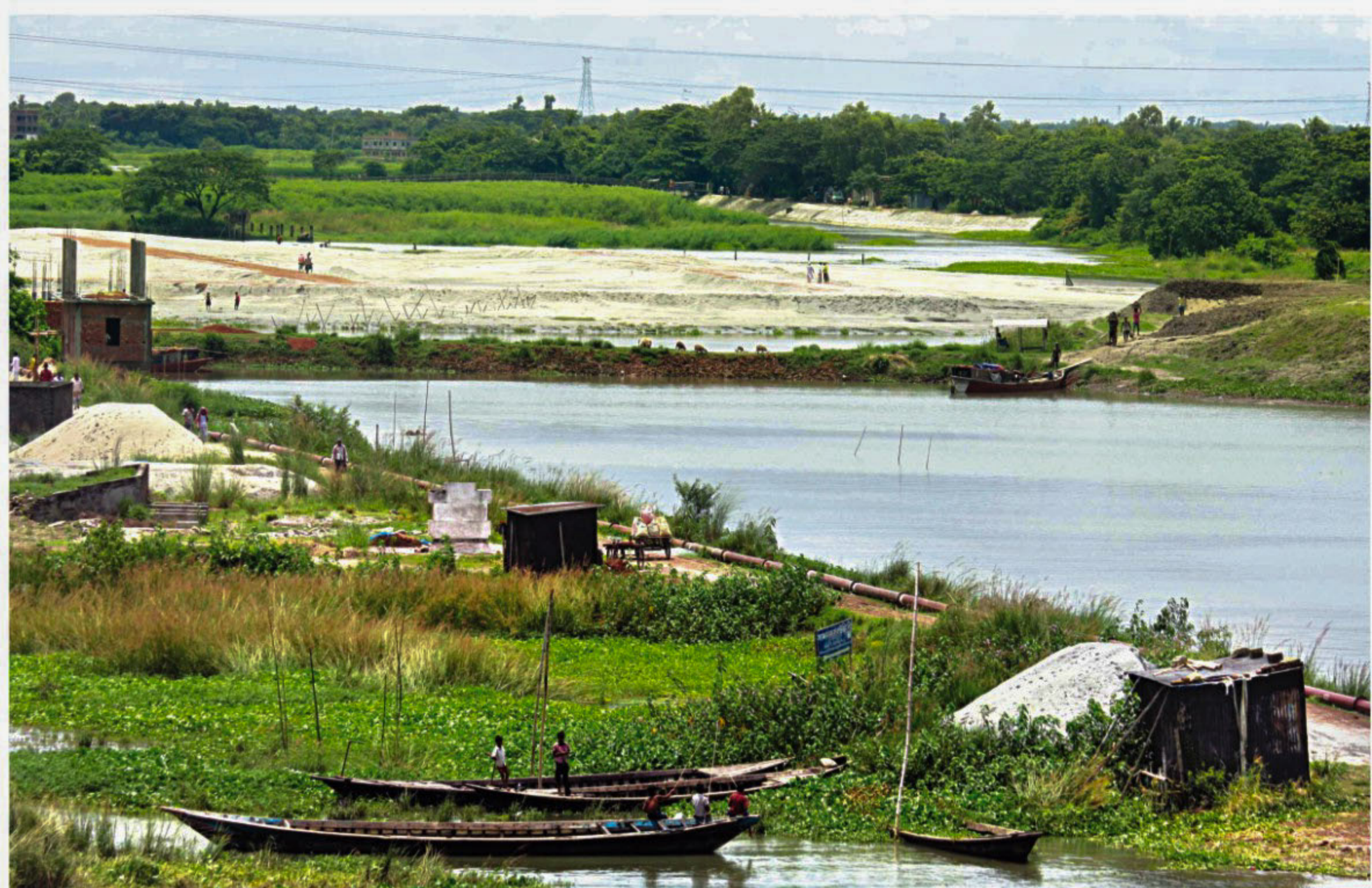
Huge pipes are being used by a real estate developer to dredge silt and fill up Atir Khal at Waaspur on the outskirts of the capital. The photo was taken earlier in the week. PHOTO: ANISUR RAHMAN
