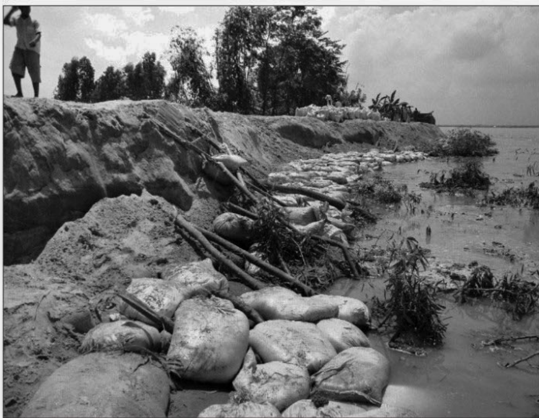
Erosion by the Teesta has damaged the dyke at Chondimari village in Aditmari upazila of Lalmonirhat district, right, the river continues devouring areas at Holdibari village in Hatibandha upazila of the district.
