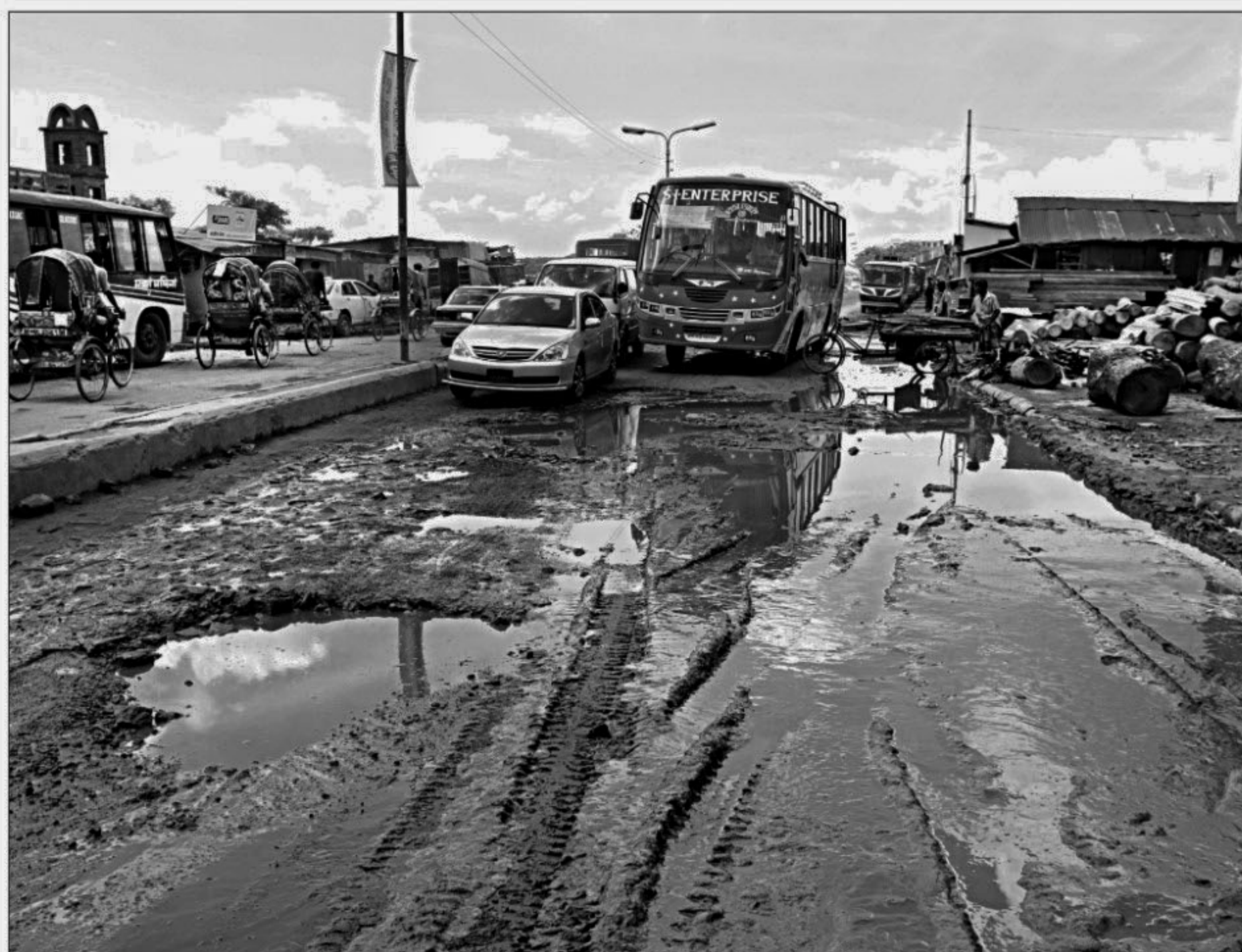
Vehicular movement on the link road from Mirpur Mazar Road to Sinnir Tek Beribadh has been disrupted for months due to the sorry state of the road.
