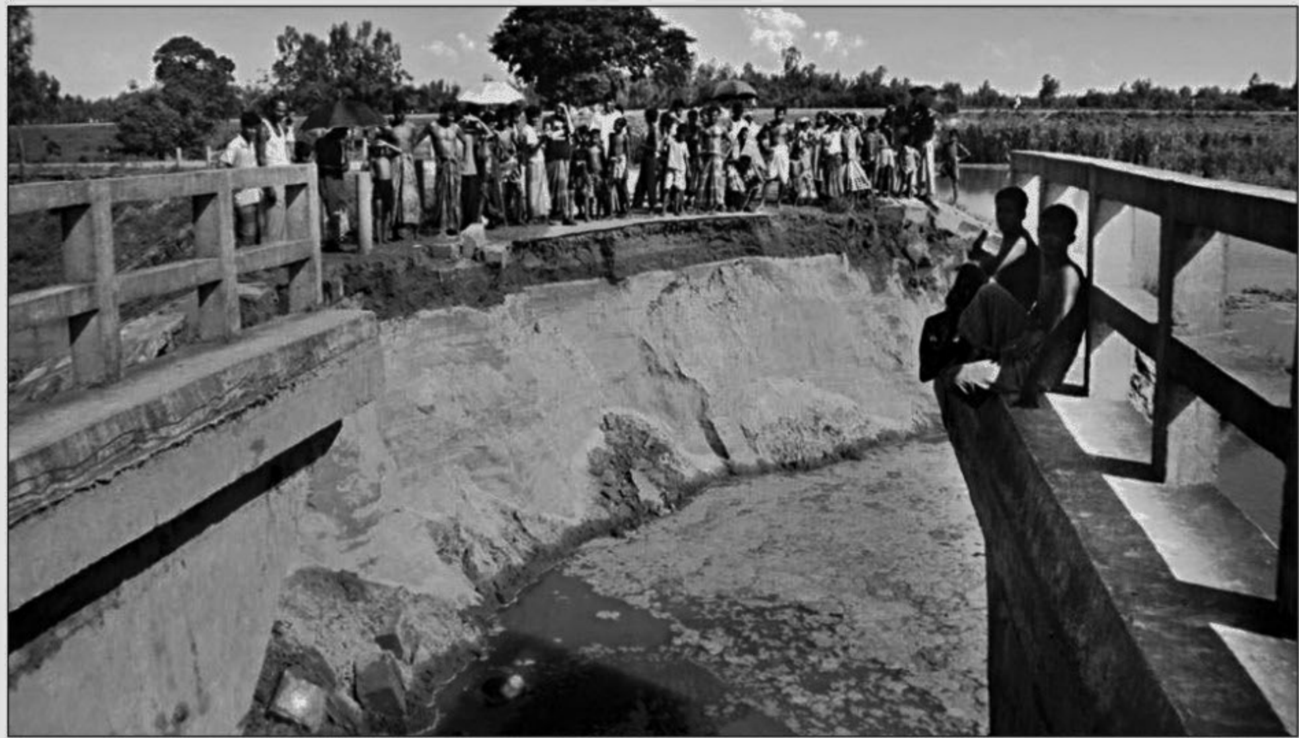
Bangali River devoured the approach road of Dewantola bridge at Mohimaganj on Sunday night, disconnecting road communication between Gobindaganj and Shaghata upazilas of Gaibandha district.
