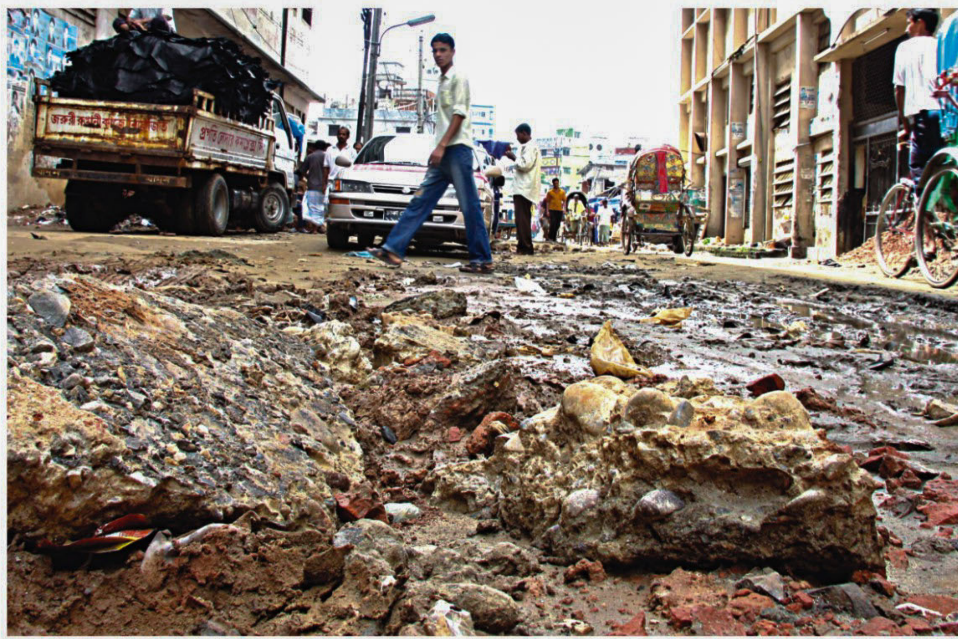
The horrible state of Tannery Road at Hazaribagh in the capital. The streets of the area are more or less in similar condition.
