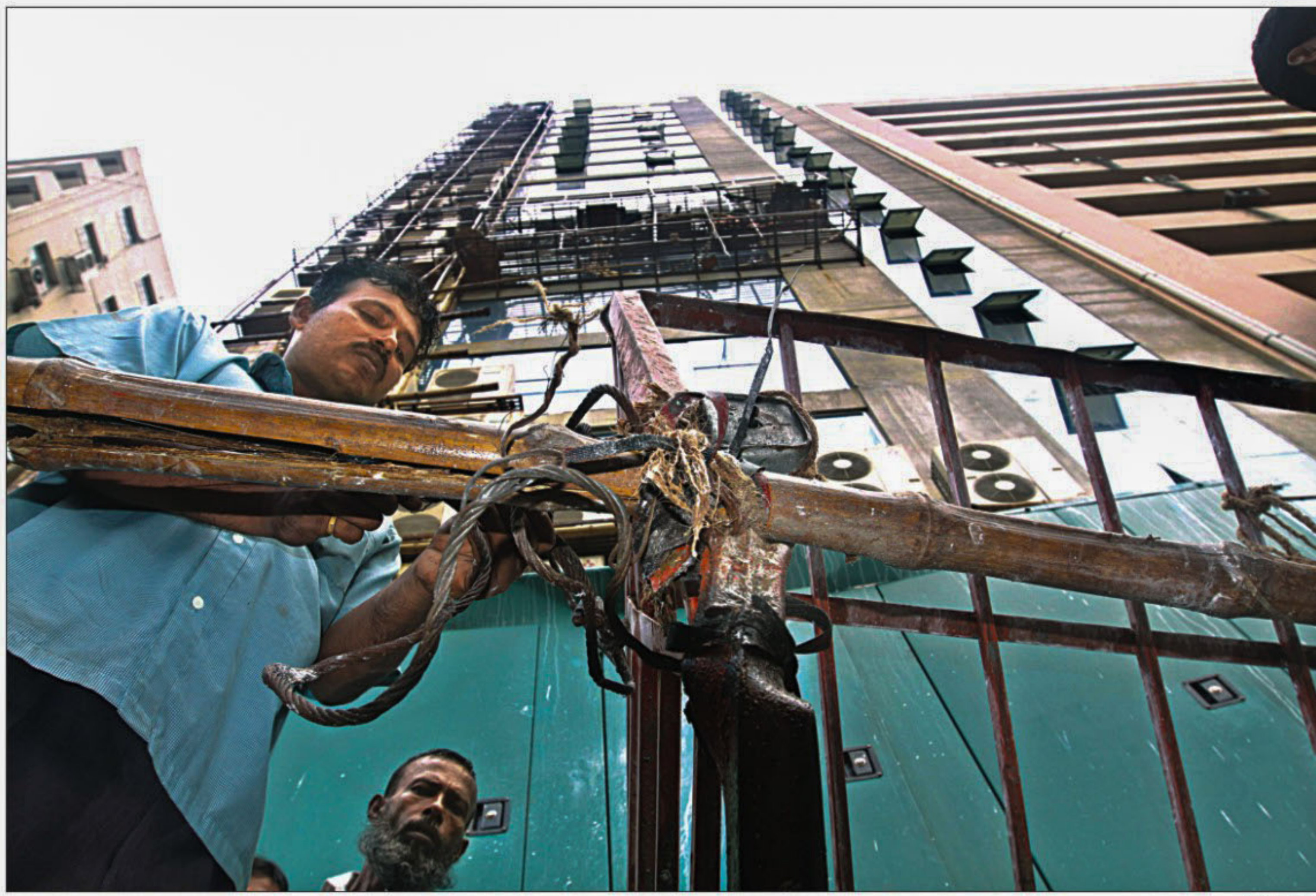
Two worker brothers died after they plunged from this high-rise at Motijheel yesterday while painting the top portion of the structure.
