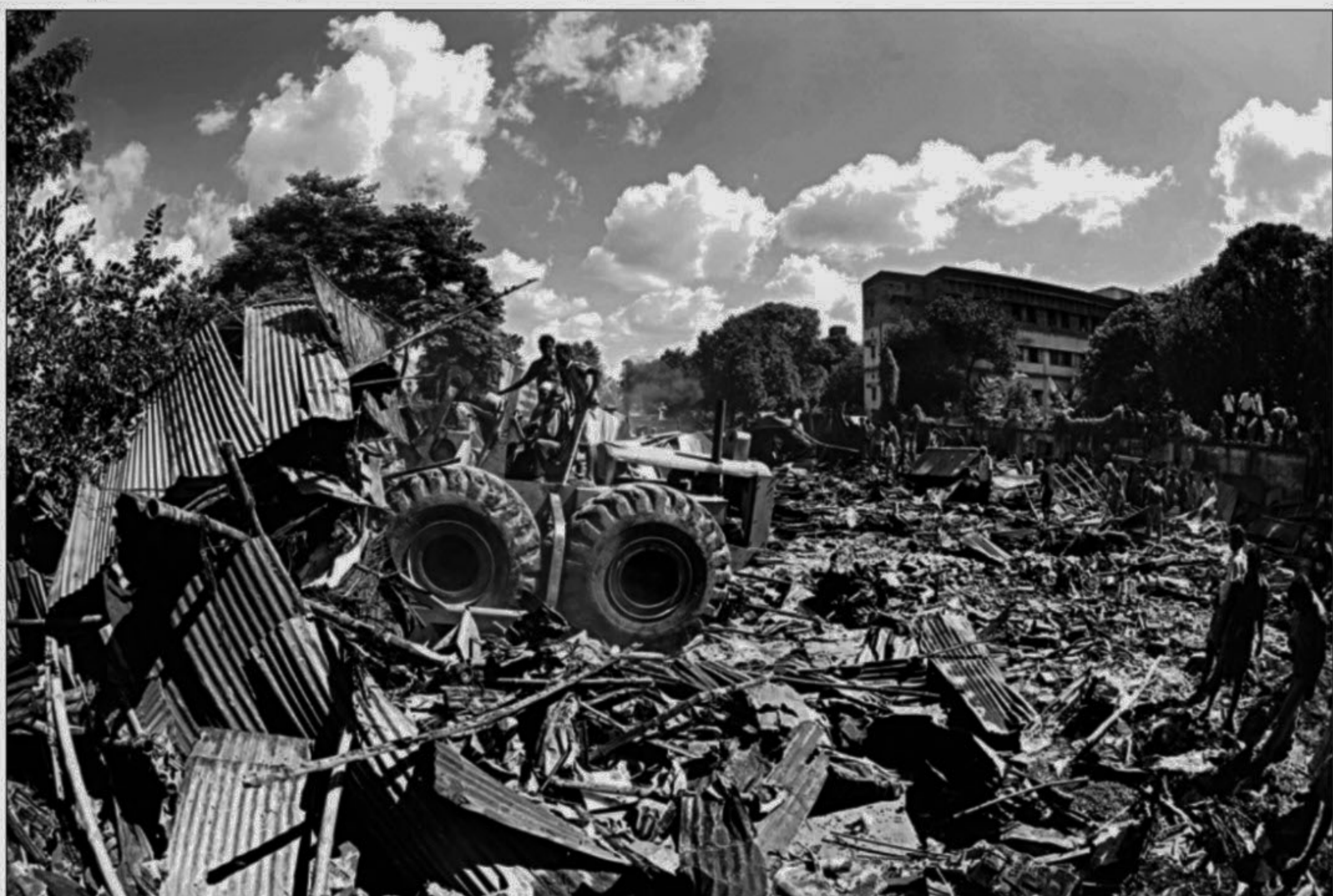
Few hours is all that was needed to destroy 2.5 acres of households.
