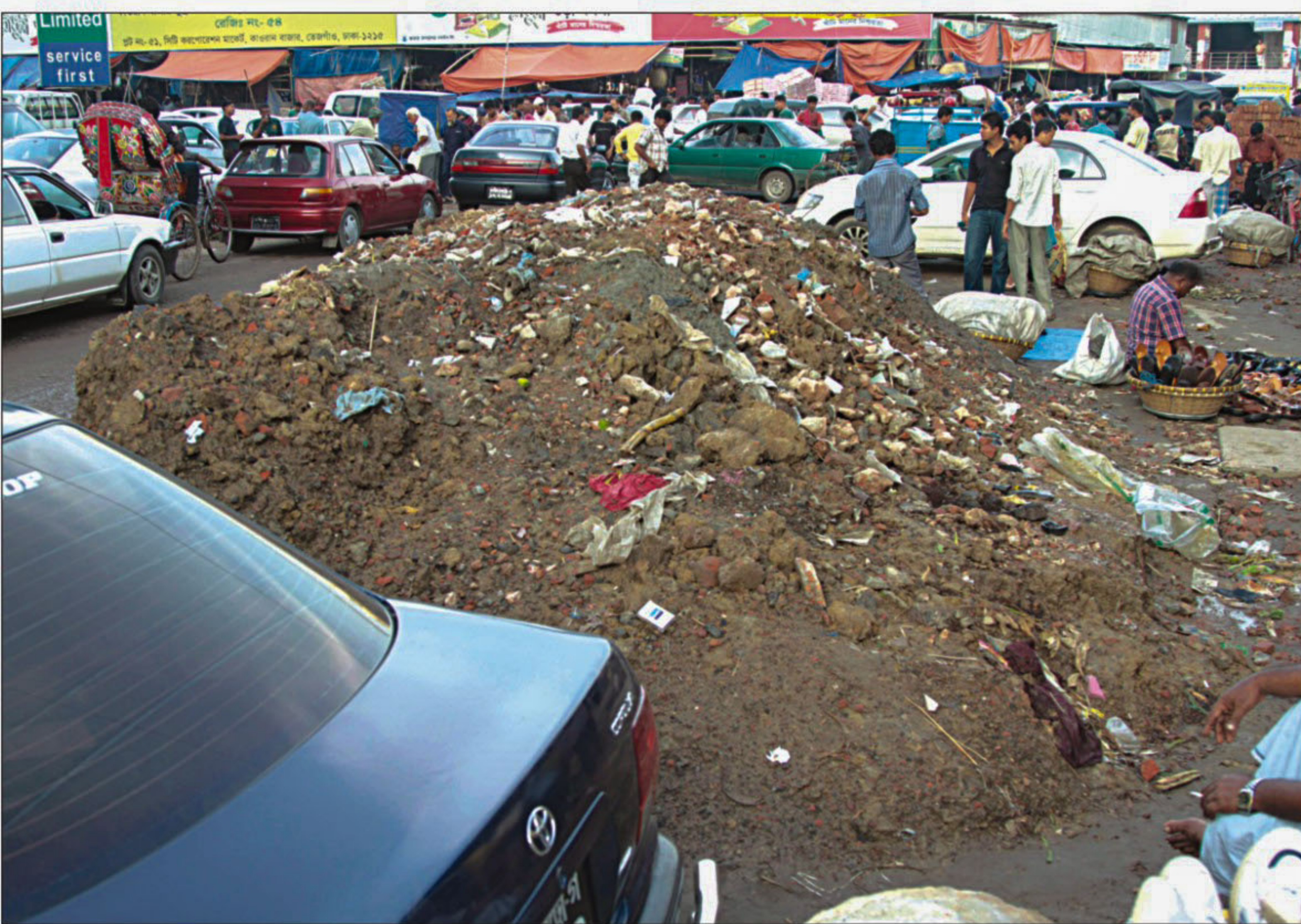
Mounds of dirt, dug up during installation of sewerage pipes, piled in front of Kawran Bazar Mosque in the city causing traffic jam as well as sufferings to the pedestrians there all day long. A week has passed since construction work has ended. The photo was taken yesterday.
