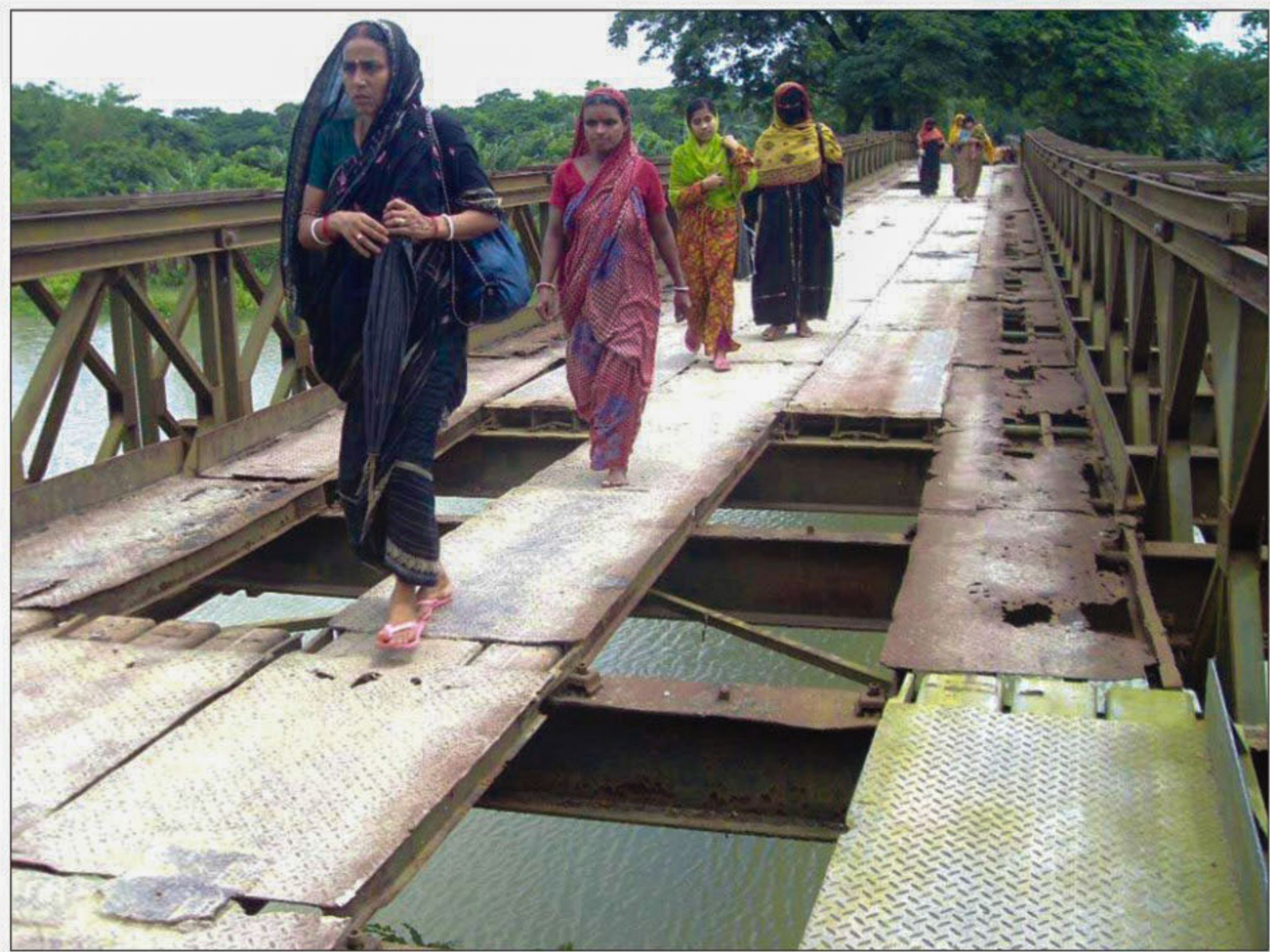
With steel plates missing at places, Telikhali Bridge on Patuakhali-Barisal Road remains highly risky for users but the authorities are showing indifference to the matter.
