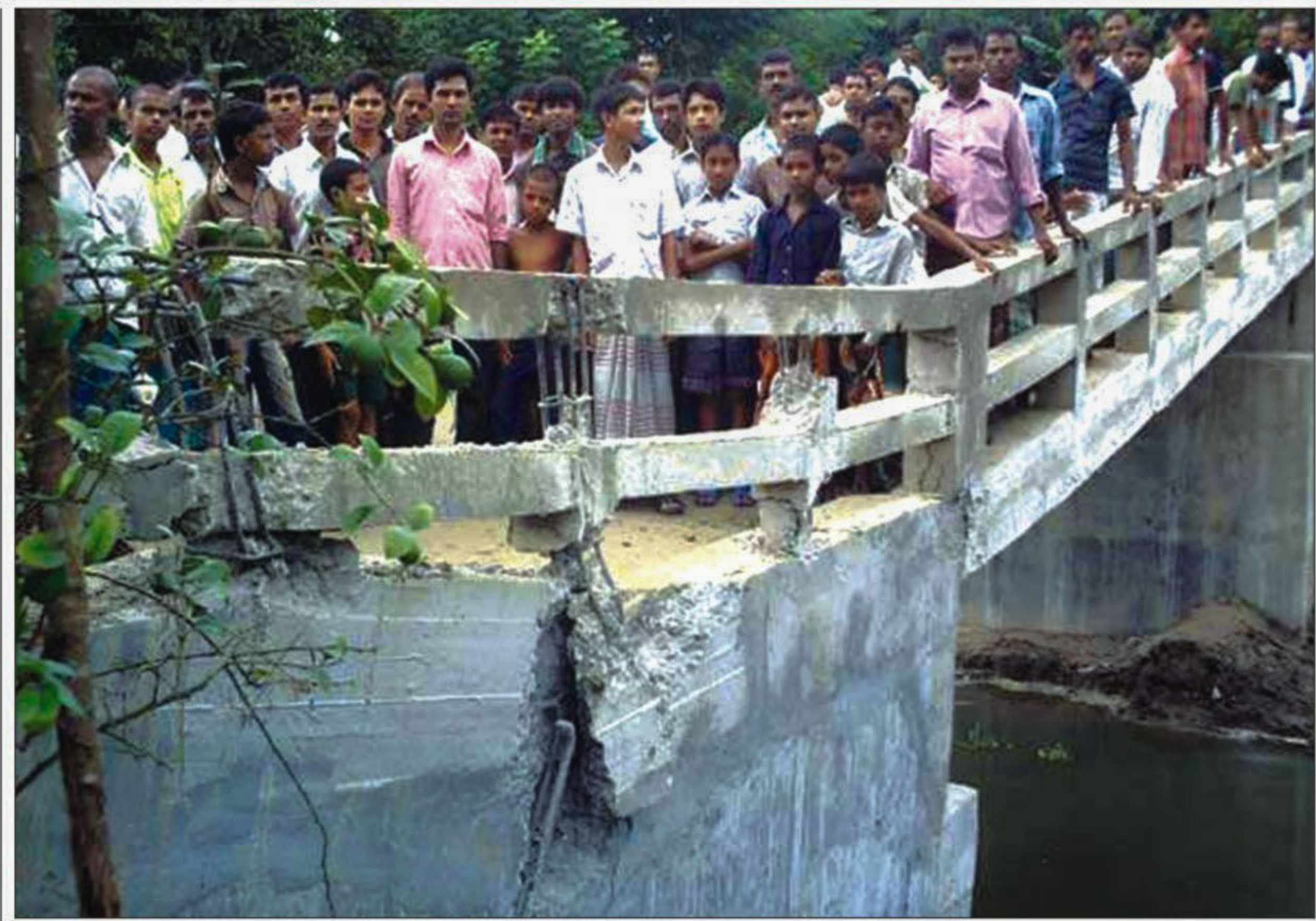
A large crack, developed on Friday shortly after removal of the temporary frame used for casting during construction of this bridge at Baraigram in Natore district, leaves it highly risky for users.
