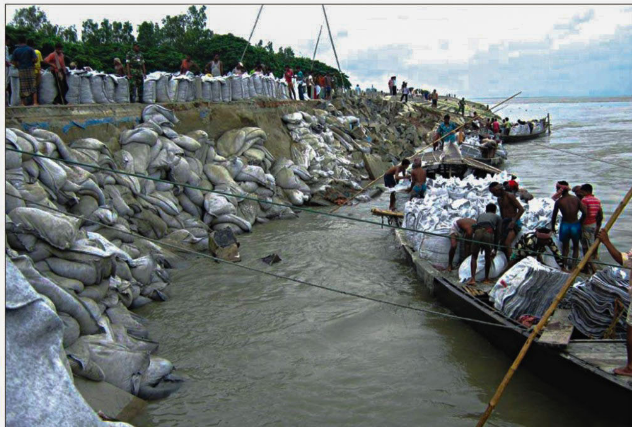
Locals join in the army efforts to protect Sirajganj Town Protection Embankment yesterday. Breaches in this embankment on the Jamuna put the district town in great danger. Story on page 13
