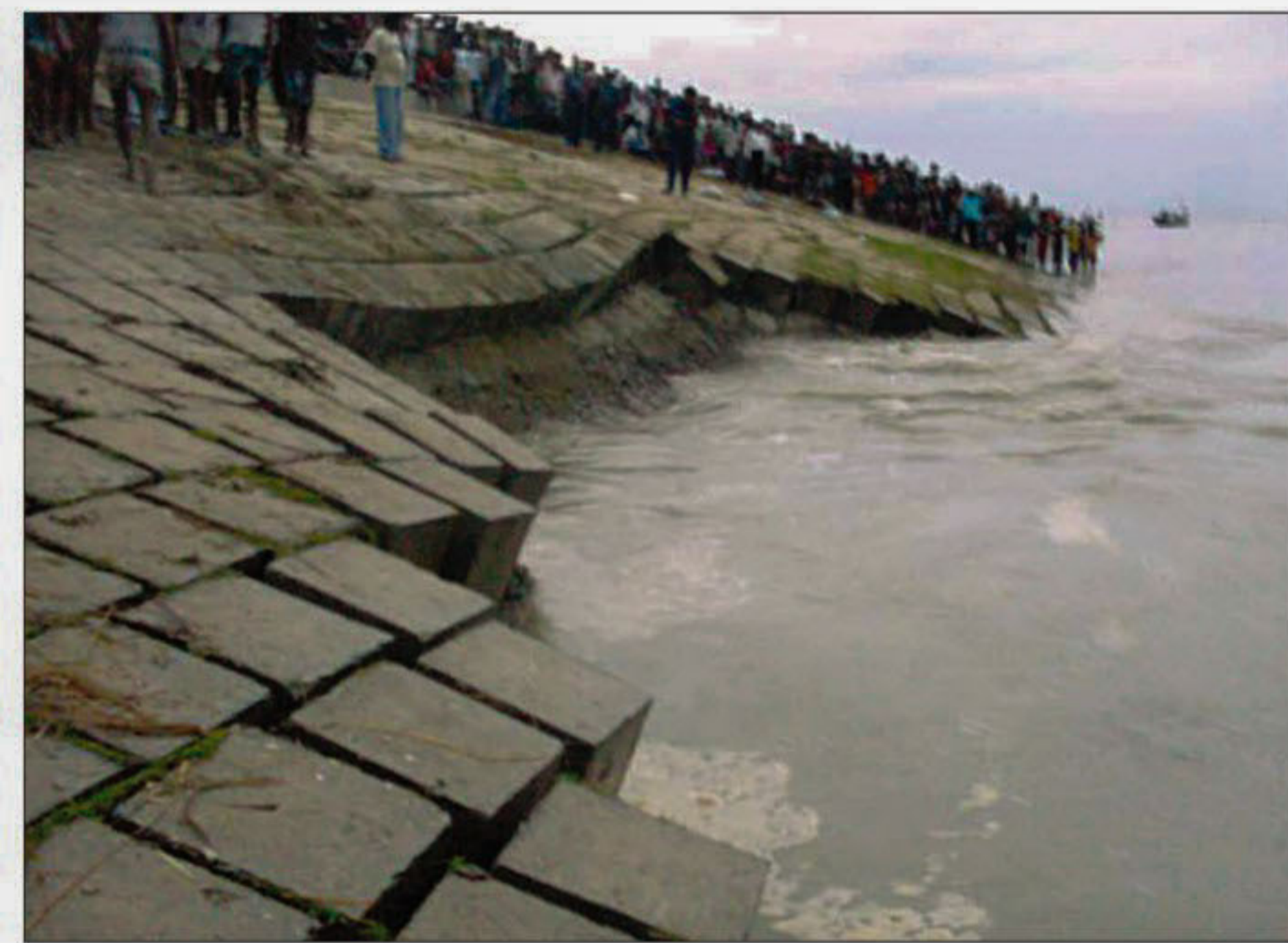
About 180-foot area of Sirajganj Town Protection Embankment goes into the Jamuna due to erosion by the turbulent river yesterday afternoon.
