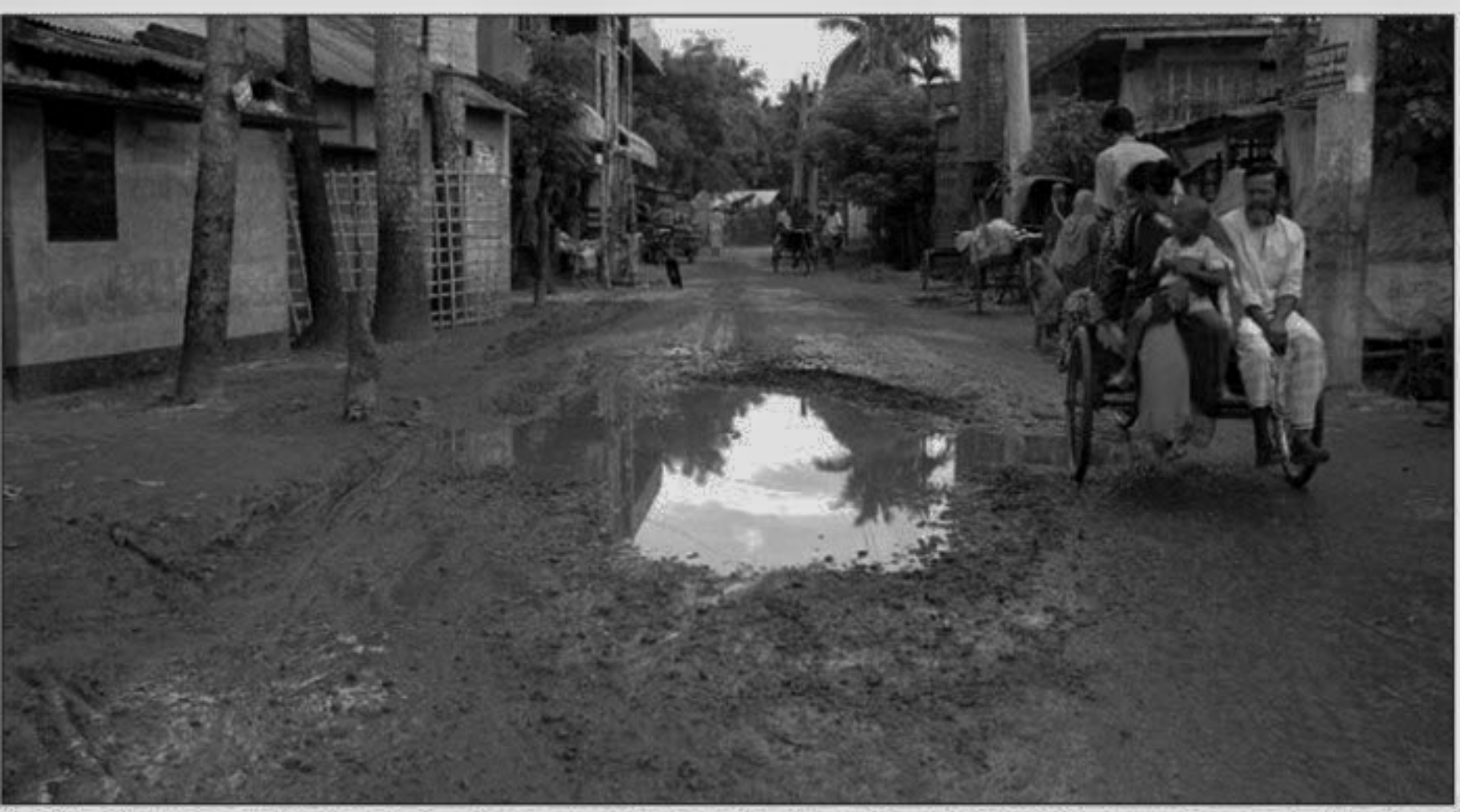
Ishak Sarak in Jessore town remains in an awfully dilapidated condition, much to the inconvenience of commuters and pedestrians.
