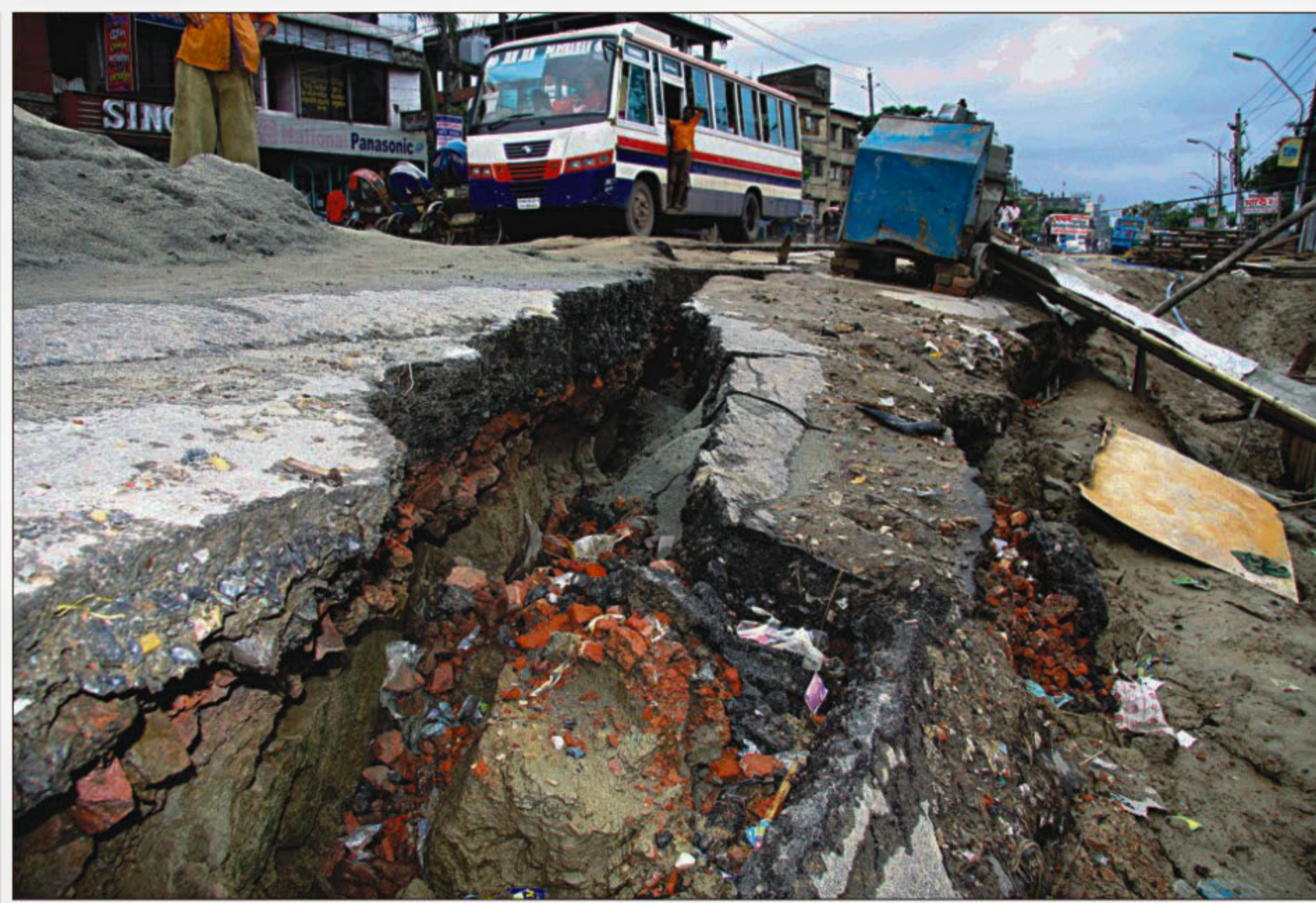
The slow pace of repair work of the road linking Jatrabari and Postagola bridge results in erosion in rainwater leaving the busy road in a dangerous state. PHOTO: ANISUR RAHMAN
