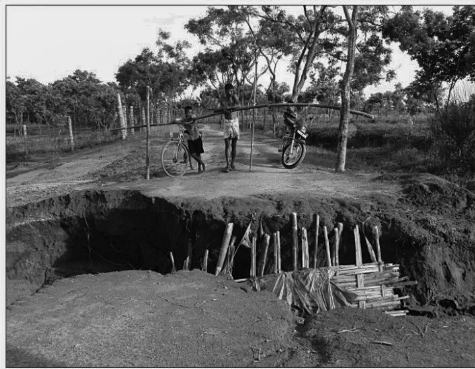
A local influential person has dug this canal across Haradighi-Roshonpur road at Roshonpur village in Tirnoi union under Tentulia upazila of Panchagarh district to drain out water from his tea garden, much to the suffering of people from several villages in the area.
