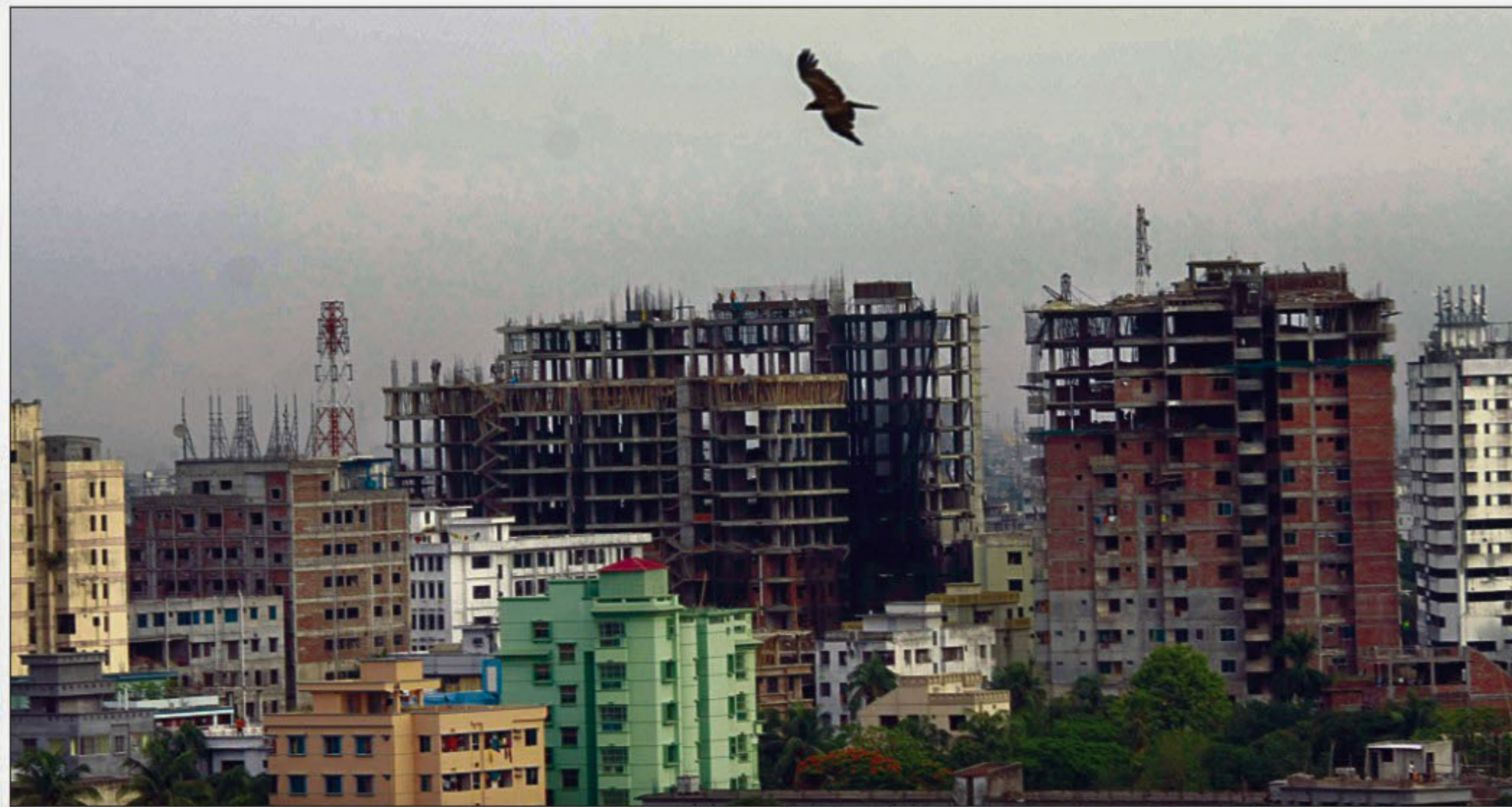
Picture shows apartments under construction. The demand for taking up such projects in the suburbs now comes to the fore to make housing affordable to the middle and lower middle-income people.
